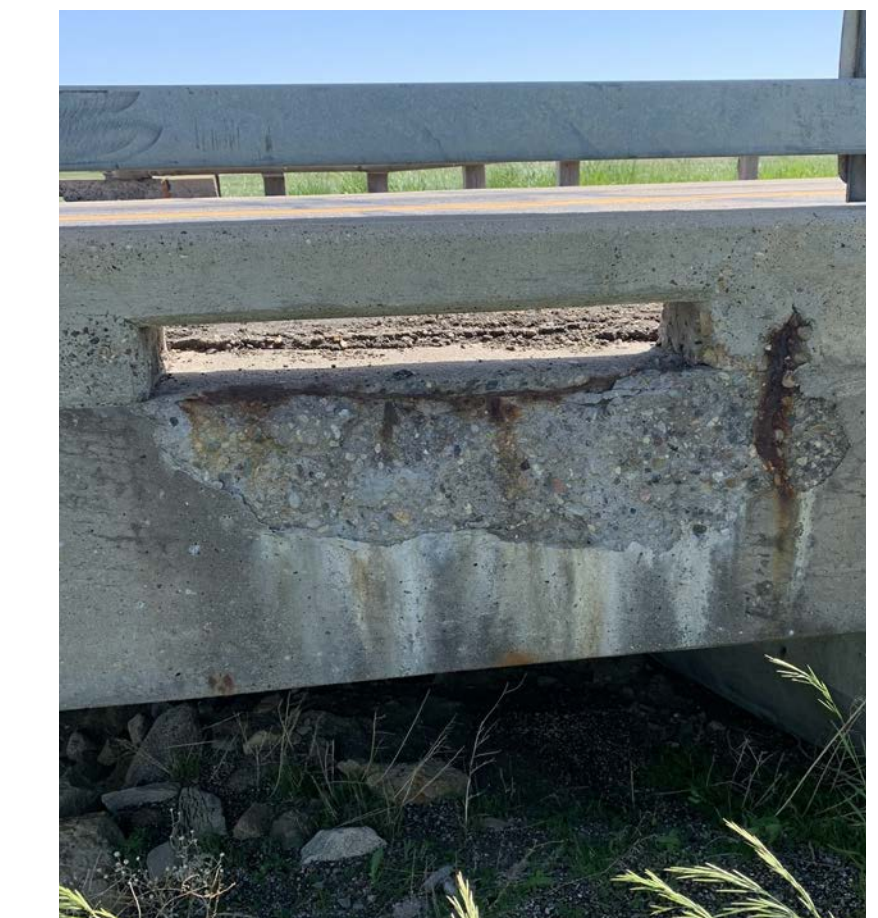
Concrete Girder Spalling with Exposed Rebar at Bridge 1806-035.070
