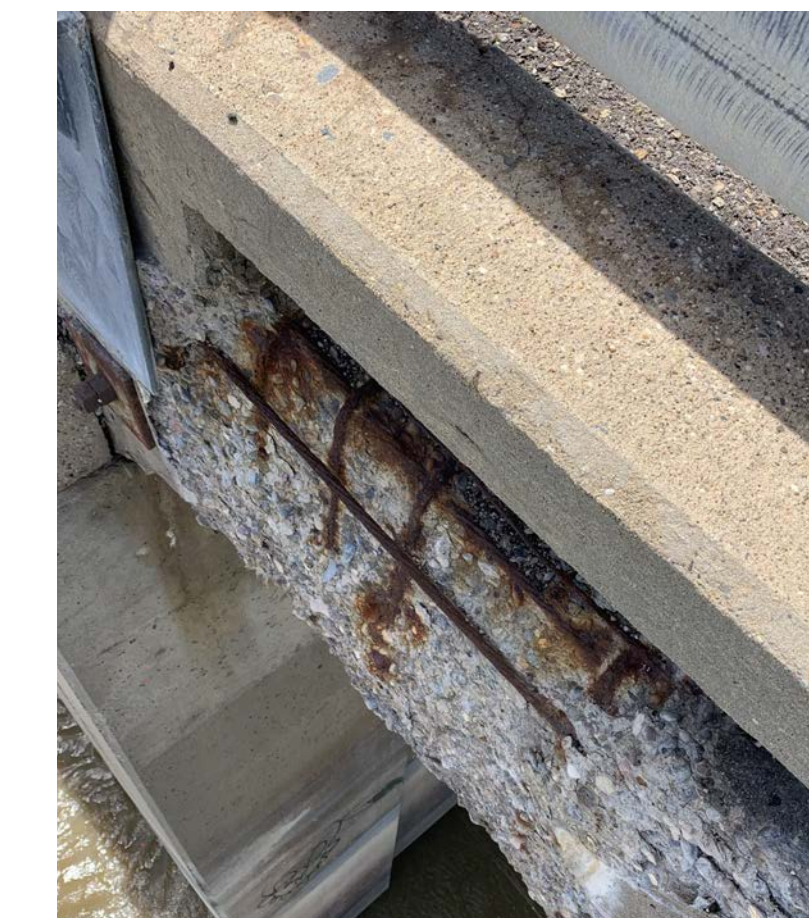
Concrete Girder Spalling with Exposed Rebar at Bridge 1806-034.280
