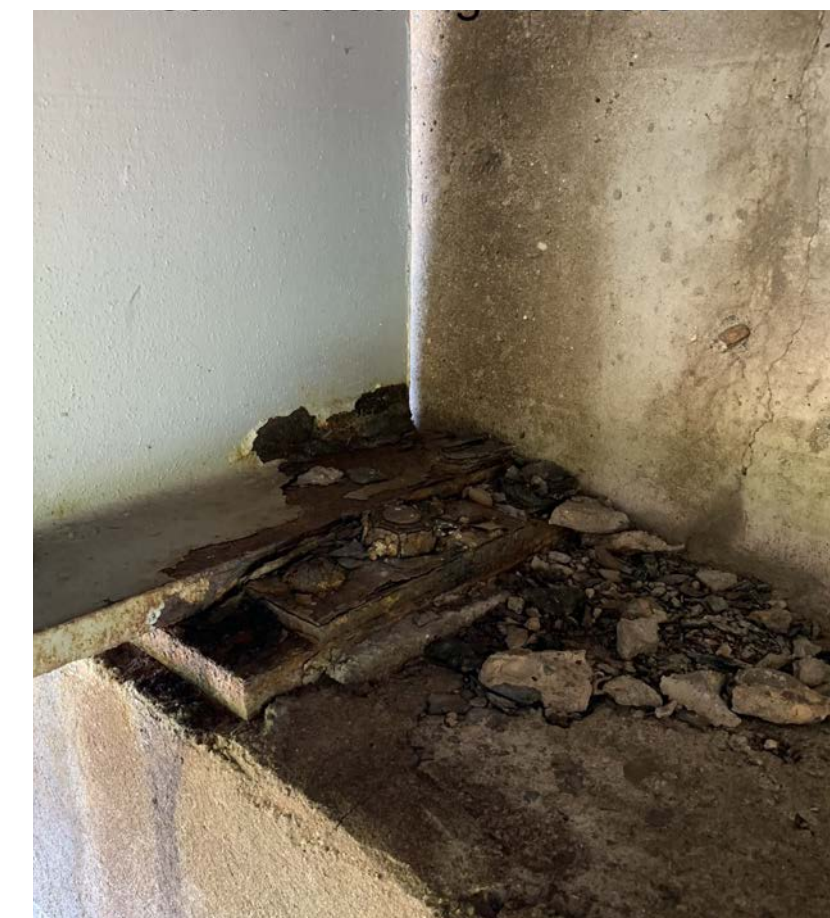
Girder/Bearing Corrosion and Abutment Cracking/Spalling at Bridge 24-000.320
