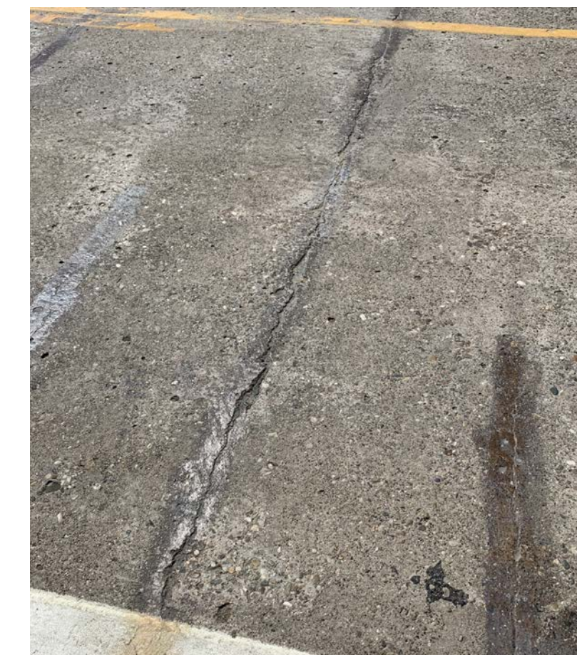
Deck Cracking at Bridge 24-000.320
