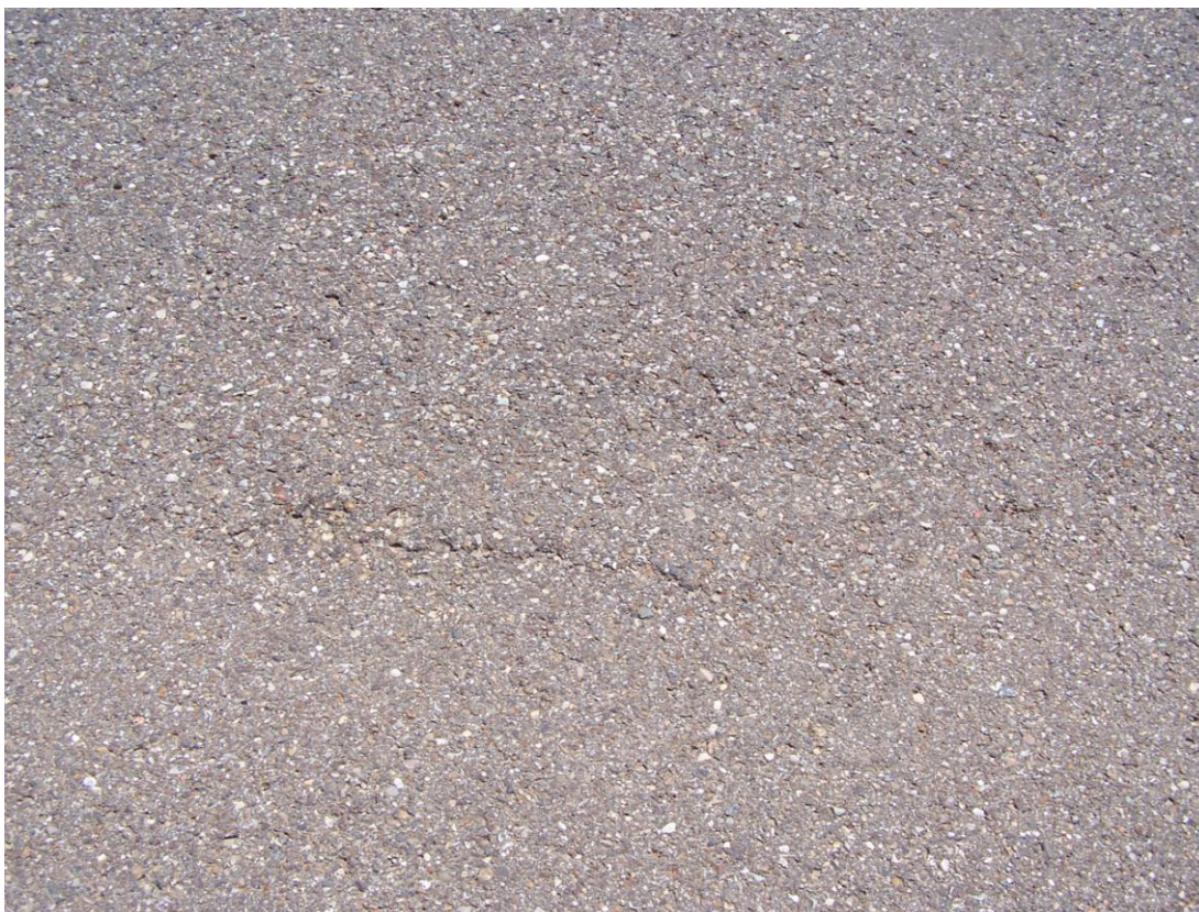
Photo 3 –Longitudinal Crack in Wheel Path with Slightly Raveled Surface.
