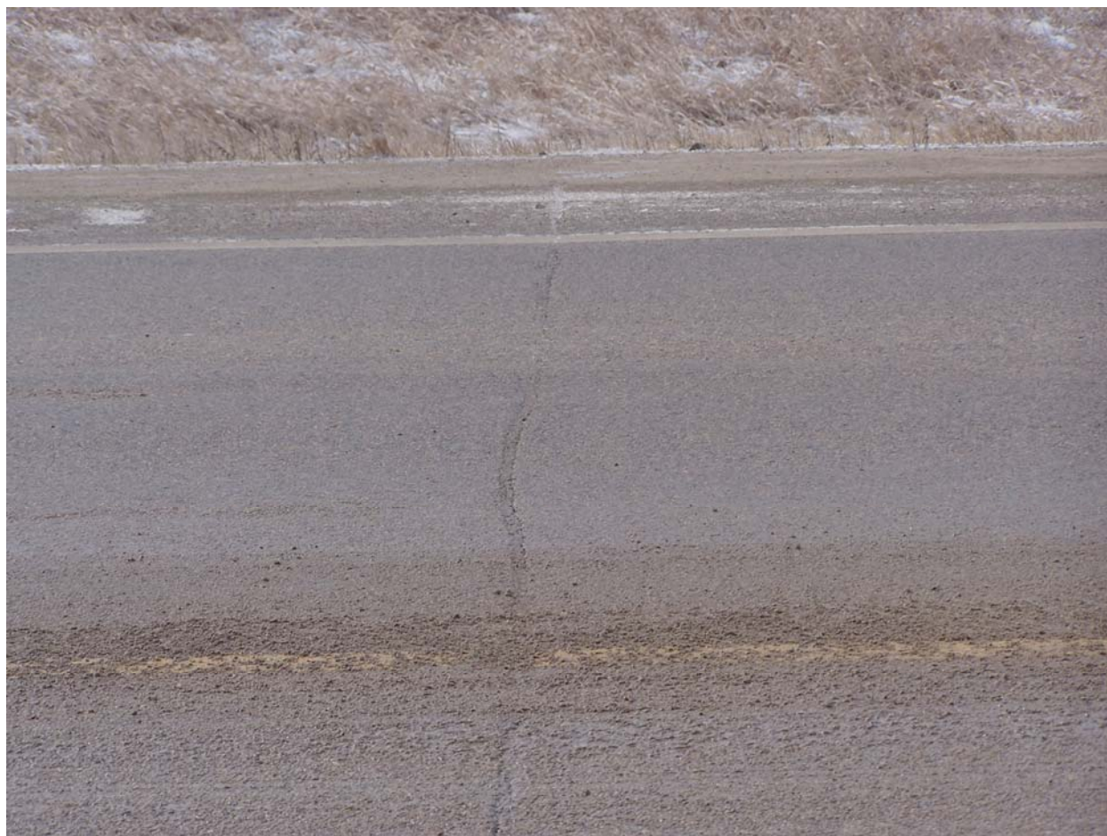
Photo 1 – Roadway shoving in wheel paths.
