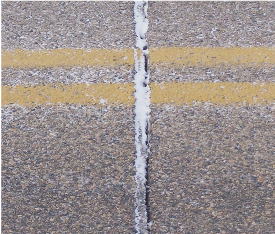
Photo 2 – Joint with sealant separating from sidewall due to adhesion failure.
