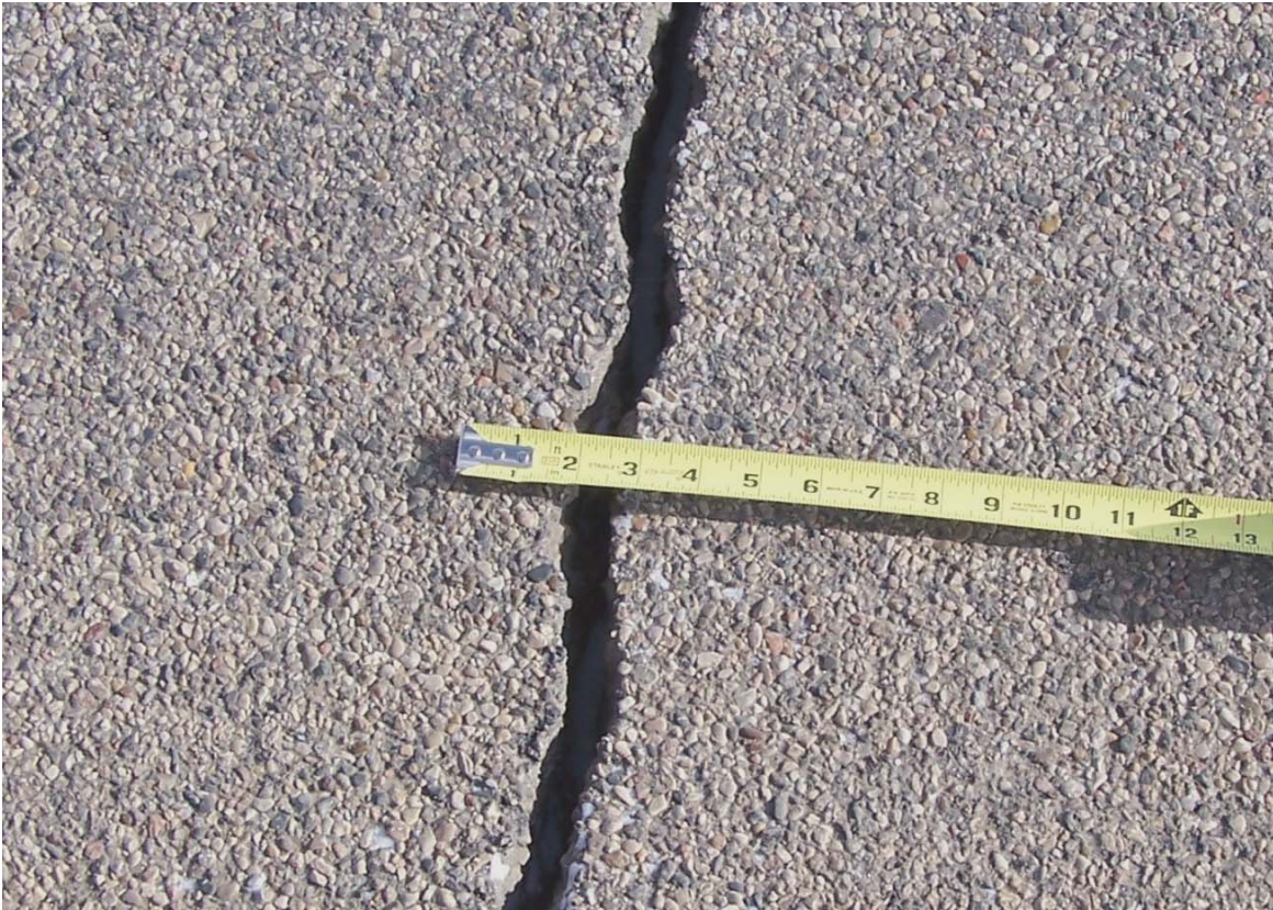
Photo 3 – An expanded random transverse crack.
