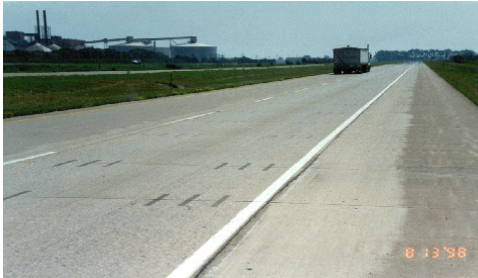
Photo 12. View of both dowel bar patch materials. Patchroc 10-60 material in foreground, followed by the 3U18 material
