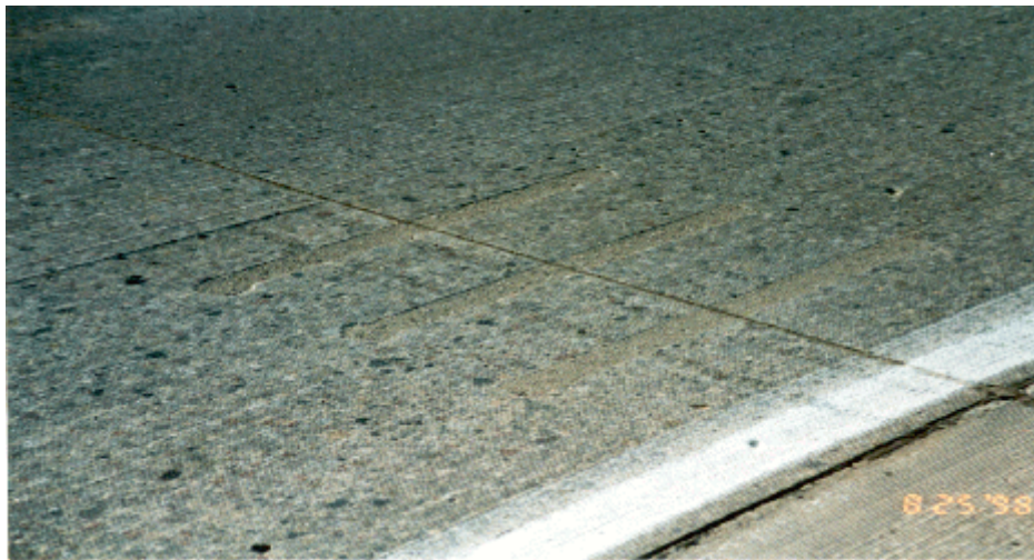
Photo 8. Close-up view of photo 7 dowel bars slots affected by mix problem
