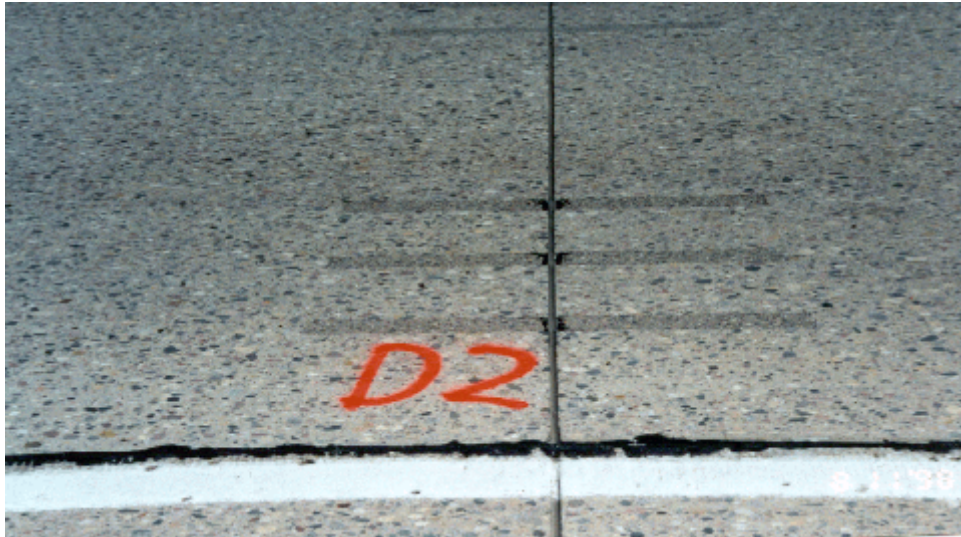
Photo 14. View of several distresses that are believed to be the result of excess silicone caulk on the slot walls prevented bonding between the existing concrete and the patching material.
