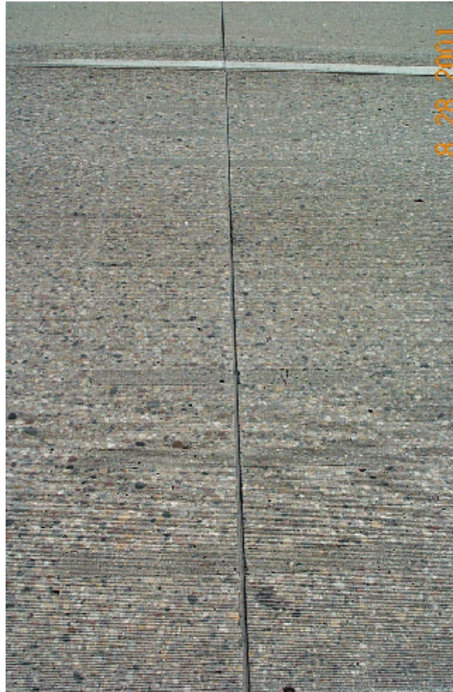
Photo 10. Typical retrofitted joint where 3U18 mix was used. Note the shrinkage crack in the 3 rd joint.
