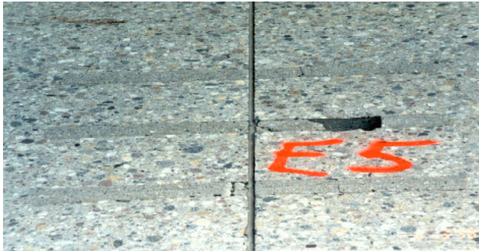
Photo 11. Dowel bar slots filled with 3U18 patch mix affected by several types of distresses including the shrinkage cracks.
