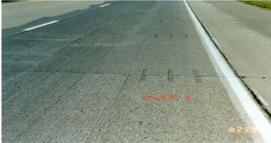
Photo 7. Dowel bars slots located in the outside wheel path of the Patchroc 10-60 section
