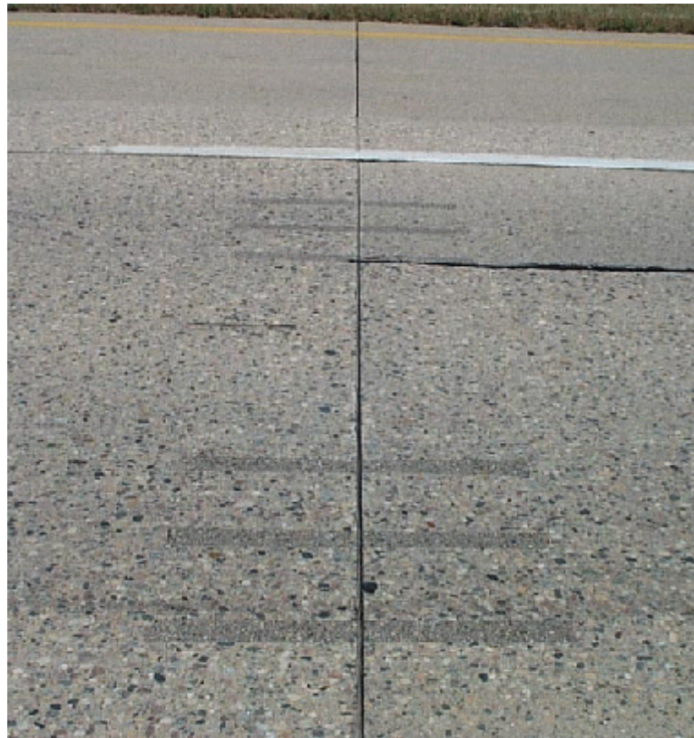
Photo 13. Typical dowel bar retrofitted joint that appears to be performing well. The longitudinal crack has not caused distress to the dowel bar patch mix.
