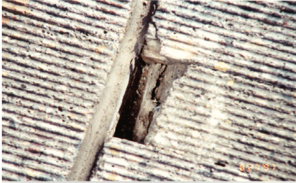
Photo 4. A view of a typical distress caused by a core board failure
