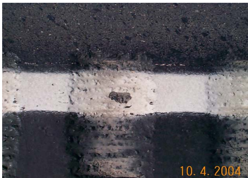
Photo 3 – Area of thick fog seal with paint flaking-off.
