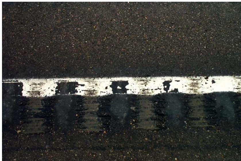
Photo 4 – A “rumble stripe” with peeling pavement marking.
