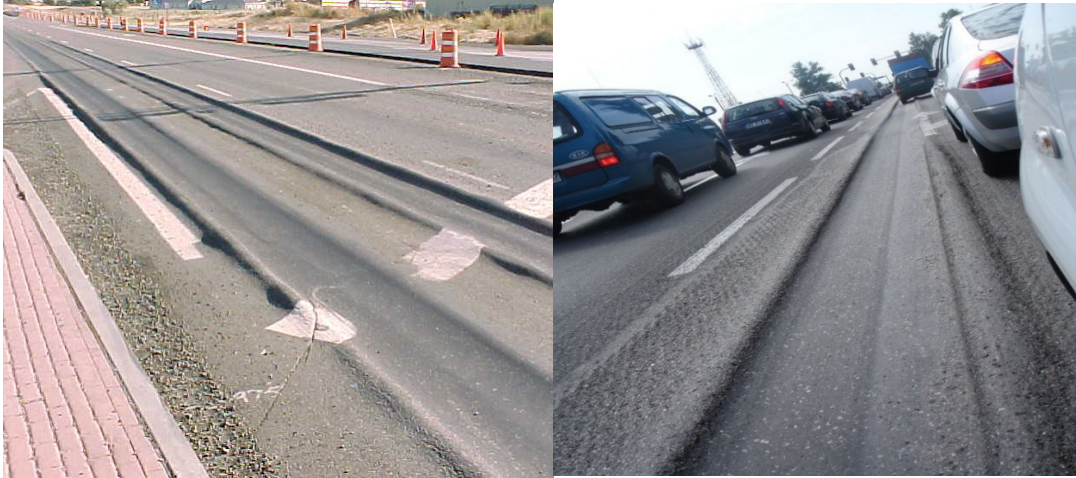
Figure 2.1: Rutting Distress in Asphalt Pavements (Wang et al., 2021).
