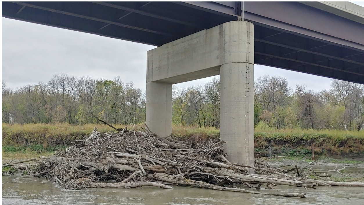
Figure 3. A log-jam formed at the upstream side of the double column central bridge pier of Highway 200 Bridge near Halstad.
