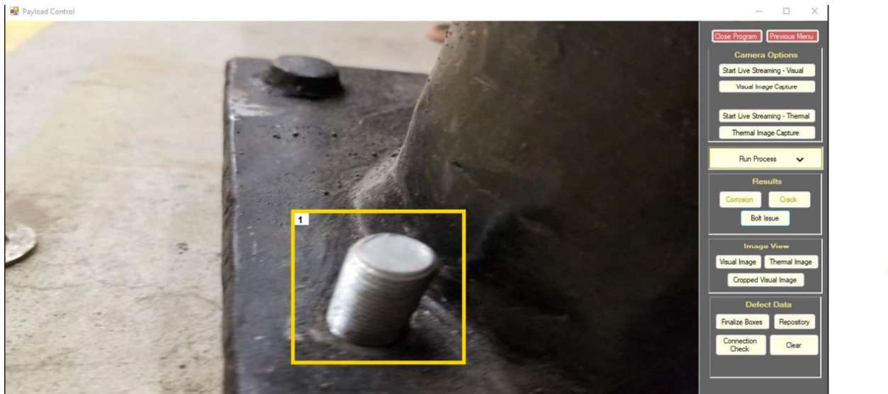
Figure 44: Bolt Defect Box Feedback
