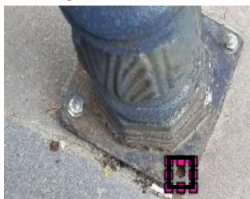
Figure 13: Structure with a missing bolt, shown by bonding box annotation
