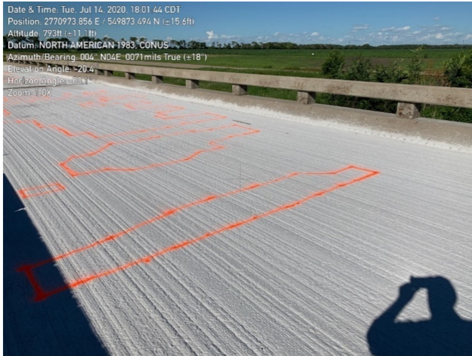
Figure 19. Park River Bridge deck markings prepared for class 2 removal after chain drag and class one removal.
