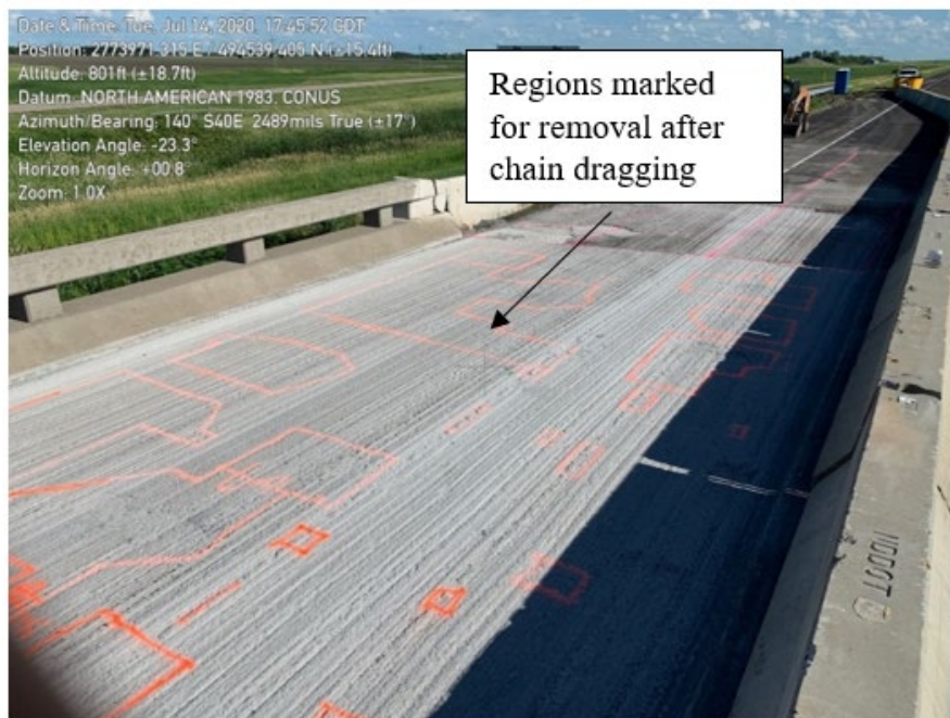
Figure 6. Forest River Bridge deck markings after chain dragging for removal of delaminated sub-surface.
