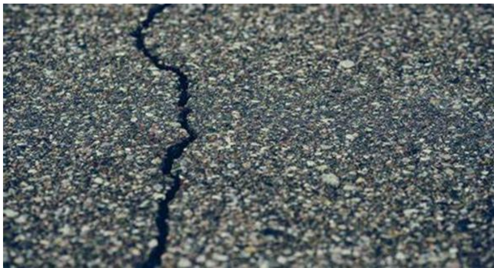
Figure 3. Images of Thermal Cracking in Asphalt Pavement (Pavement Interactive, 2009)
