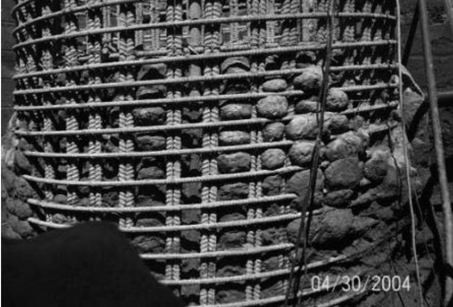
Figure 5: Drilled shaft not encapsulated by concrete [19]
