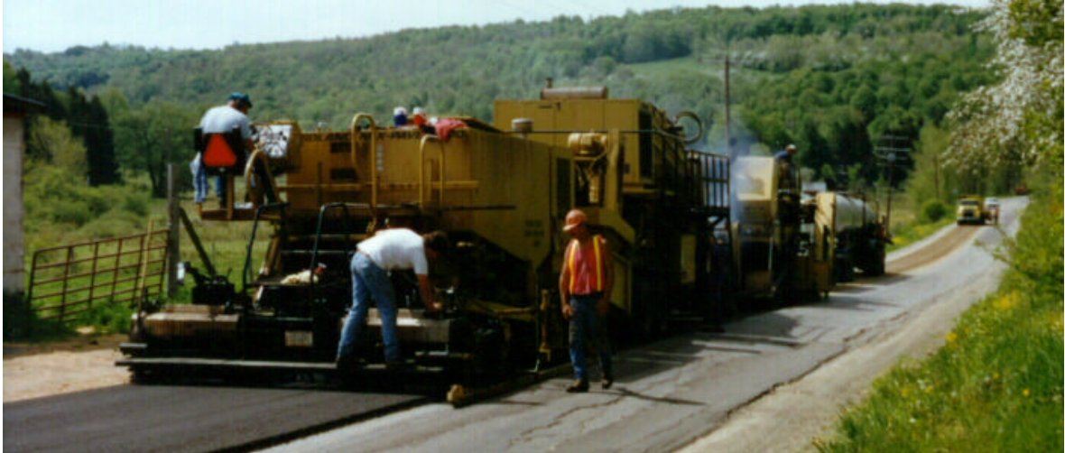
Figure 3.11. A multi-unit recycling train in action.
