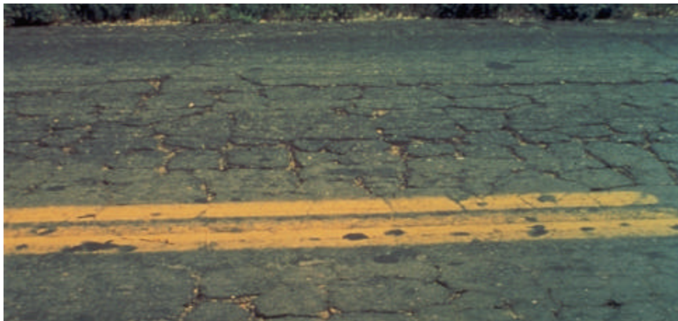
Figure 4.2. Condition of US 64 (in 1984) before CIR construction.
