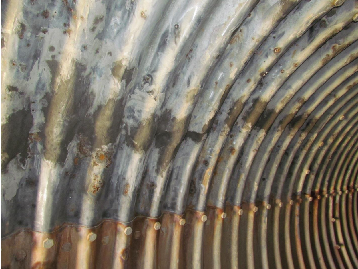
Photo 4 – Deteriorated holes filled with mortar.
