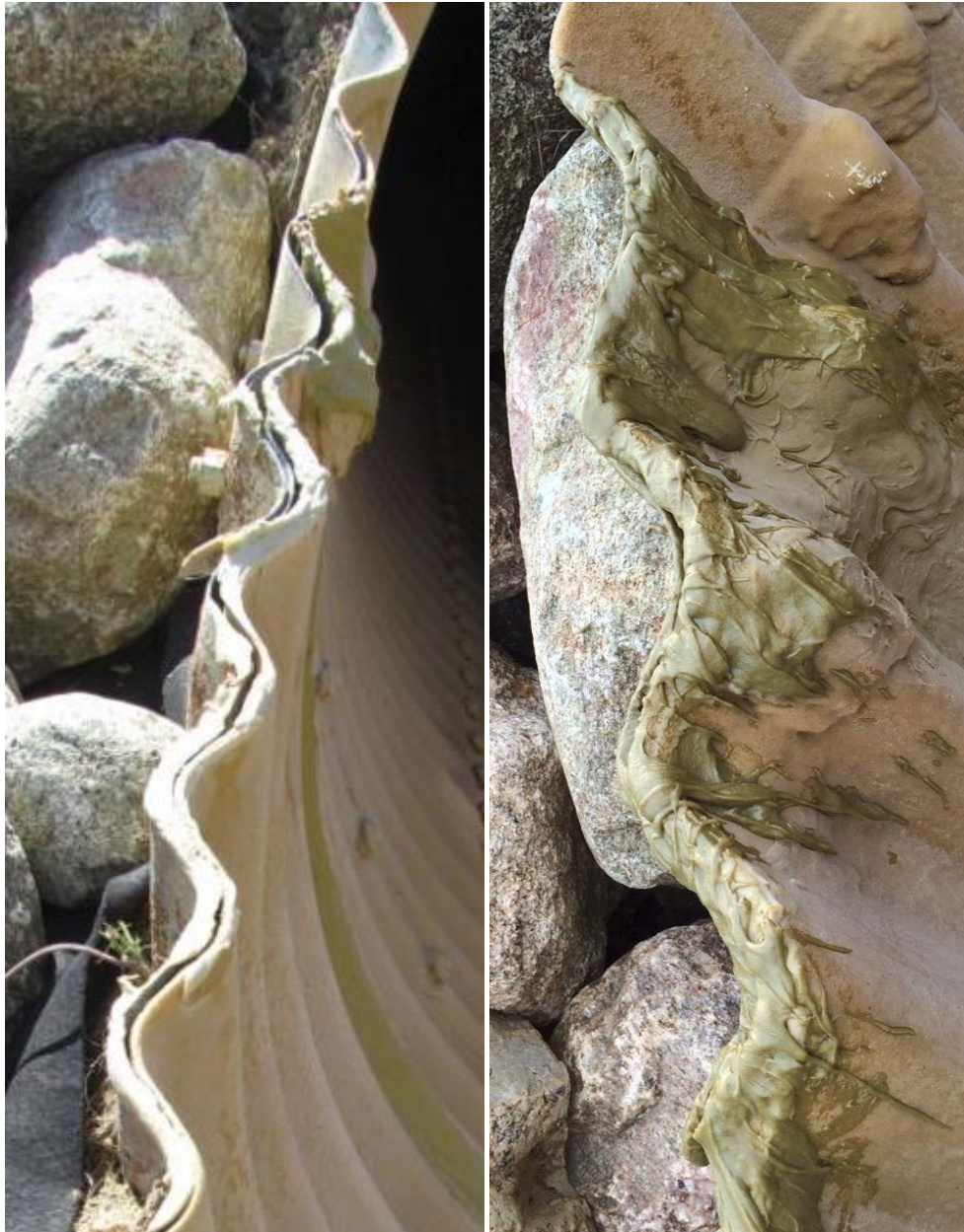
Photo 17 – Delamination between edge of end section and Spraywall liner.
