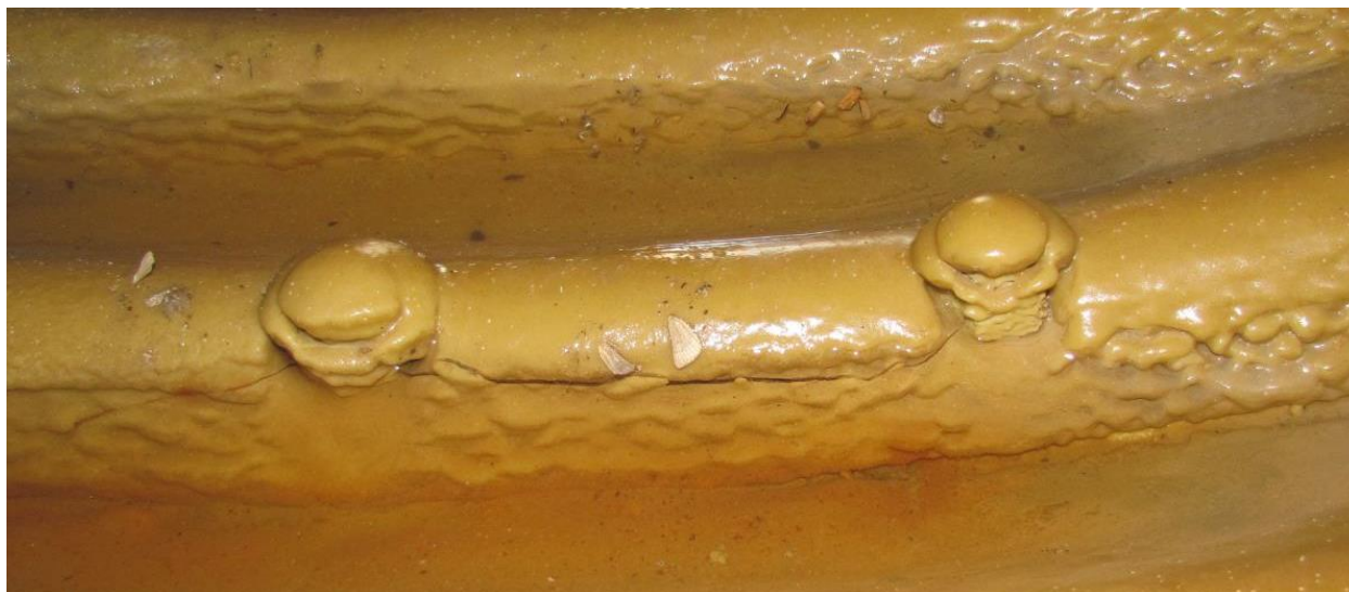
Photo 18 – Crack on the bottom of pipe 50' in from end of pipe.
