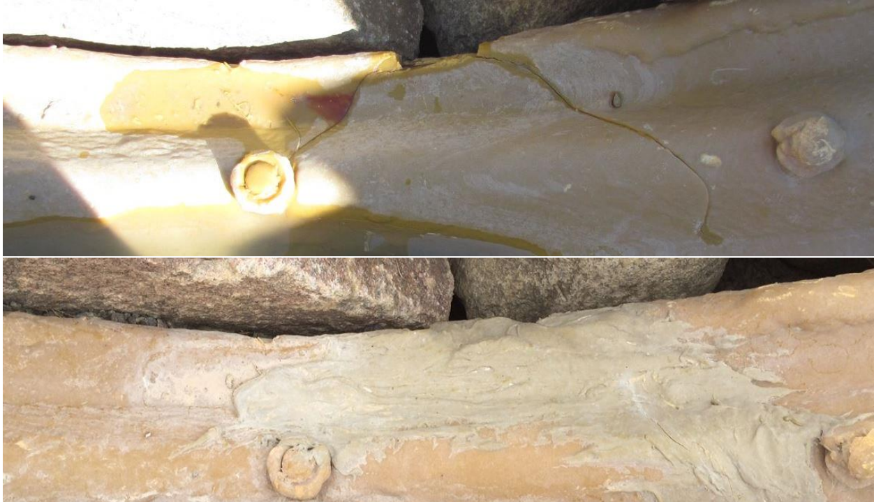
Photo 14 – A crack on the bottom edge of the end section. It appears the installation of riprap caused the damage.
