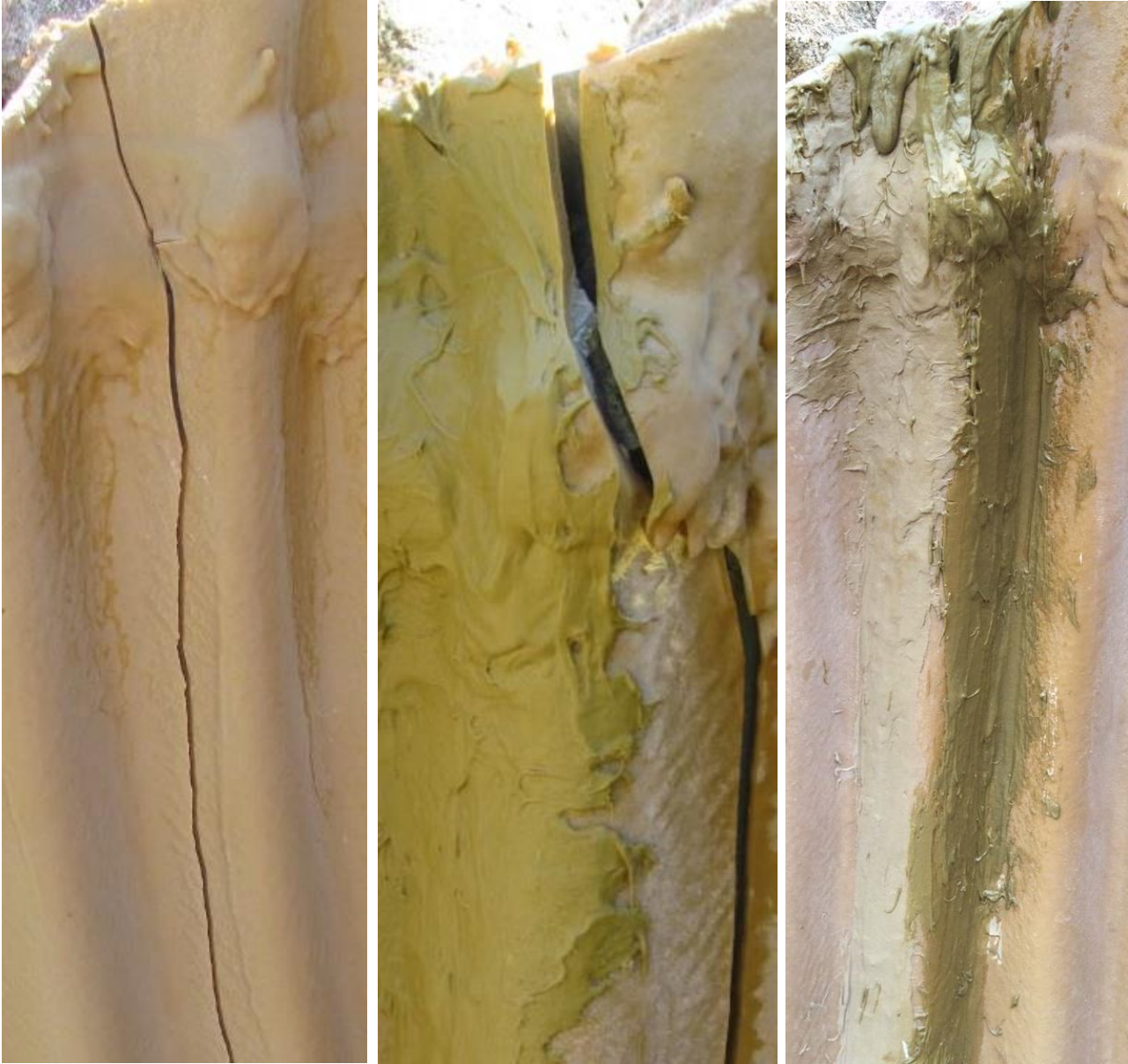
Photo 16 - A crack at the side edge of the end section before and after the repair. After the repair was complete, another crack formed parallel next the repaired crack. The new crack was repaired Subsurface.
