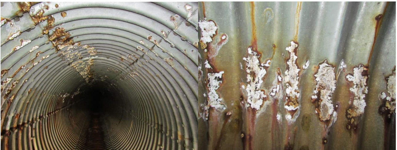
Photo 1 – Deterioration and corrosion of steel pipe.
