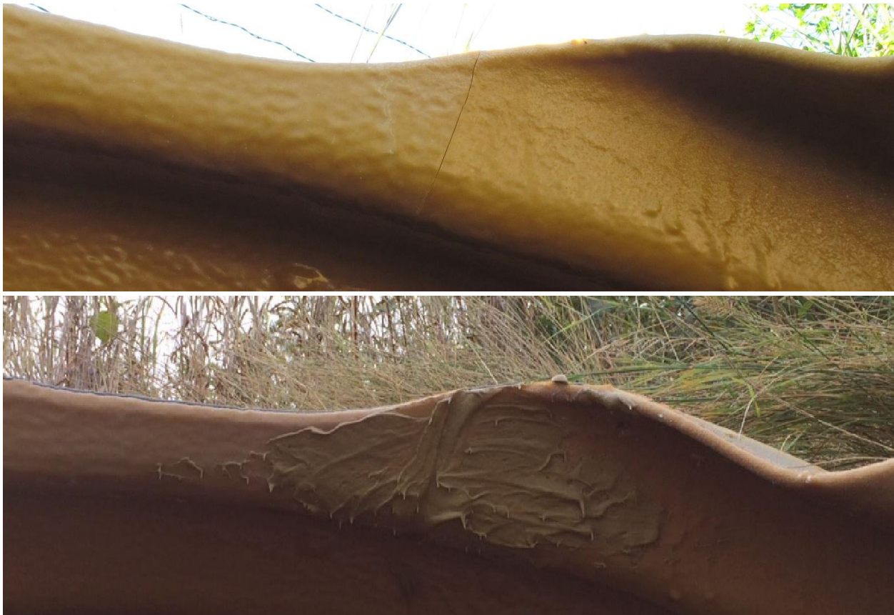
Photo 15 – A crack at the top edge of the end section before and after the repair.
