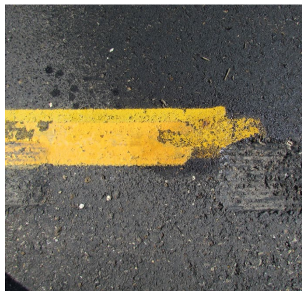
Photo 11 – After cleaning, temporary paint visible underneath, indicating that the black material is fog seal.
