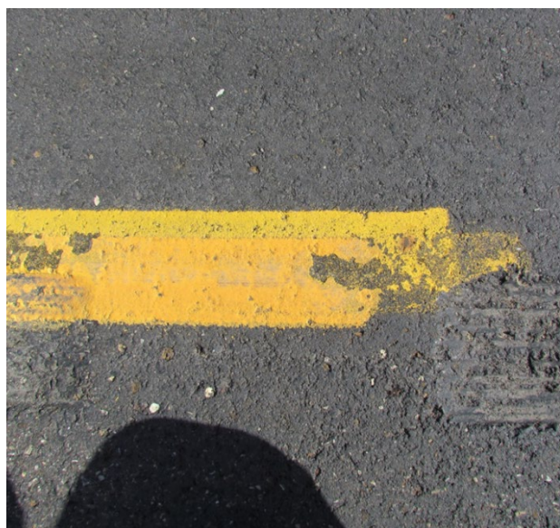
Photo 10 – Delaminated areas appear to show HMA Underneath.
