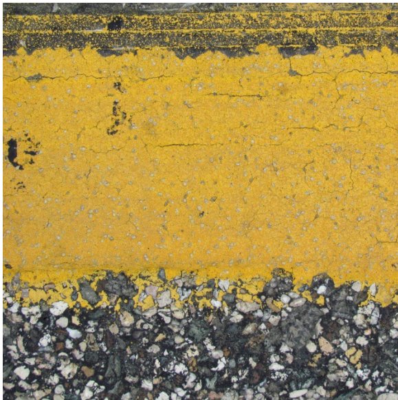
Photo 3 – Cracks in Water-based Marking
