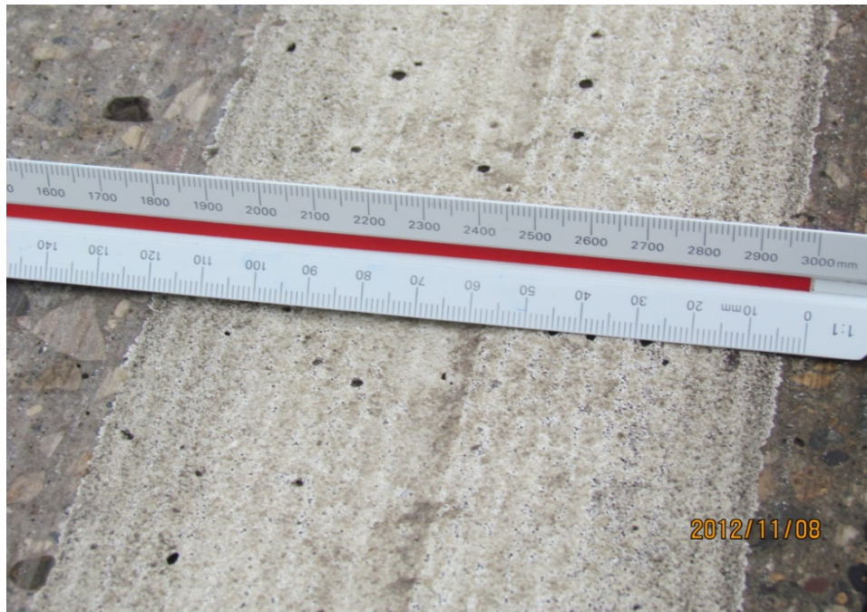
Photo 2: Surface applied epoxy placed on top of the ridge from two adjacent passes of the diamond grinder.
