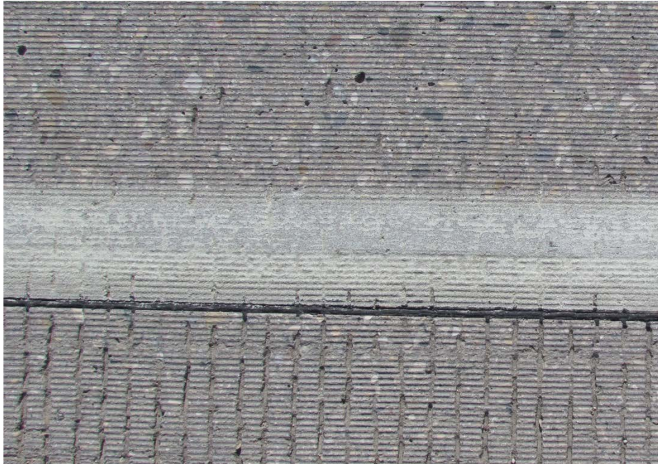
Photo 3: Surface applied epoxy with standard glass beads after 3 winters.
