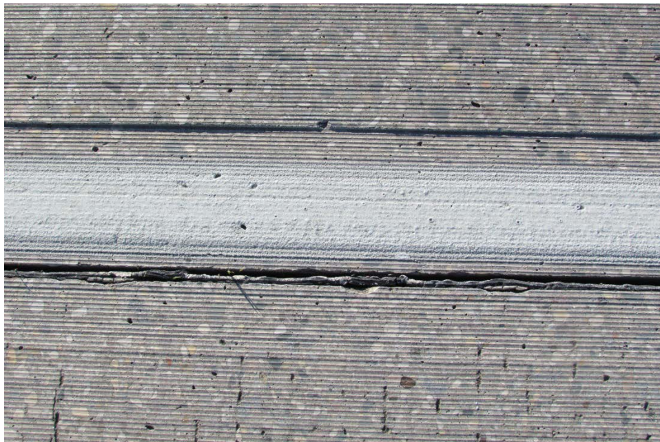
Photo 1: Ridge from two adjacent passes of the diamond grinder above the surface applied epoxy.
