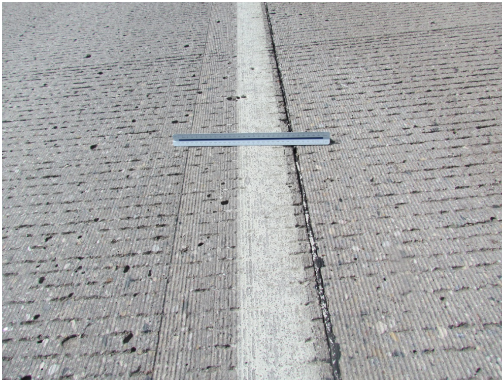
Segment 3B – NB White Surface applied Epoxy with 3M AW Elements – RP 147
