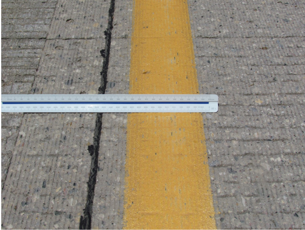
Segment 3A - NB Yellow Surface applied Epoxy with Standard Glass Beads – RP 145
