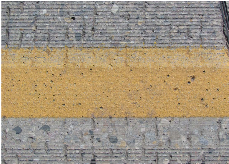
Photo 9: Grooved epoxy with improper placement after 3 winters.
