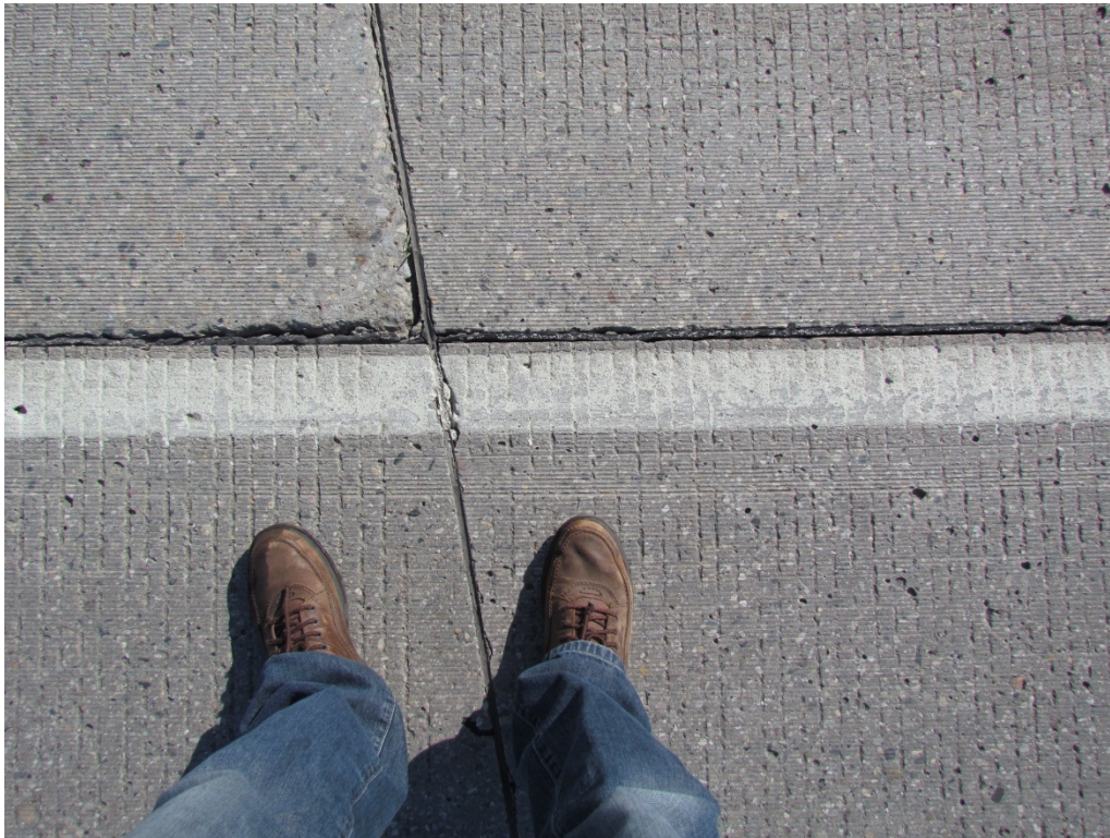
Segment 3B - NB White Surface applied Epoxy with 3M AW Elements – RP 147
