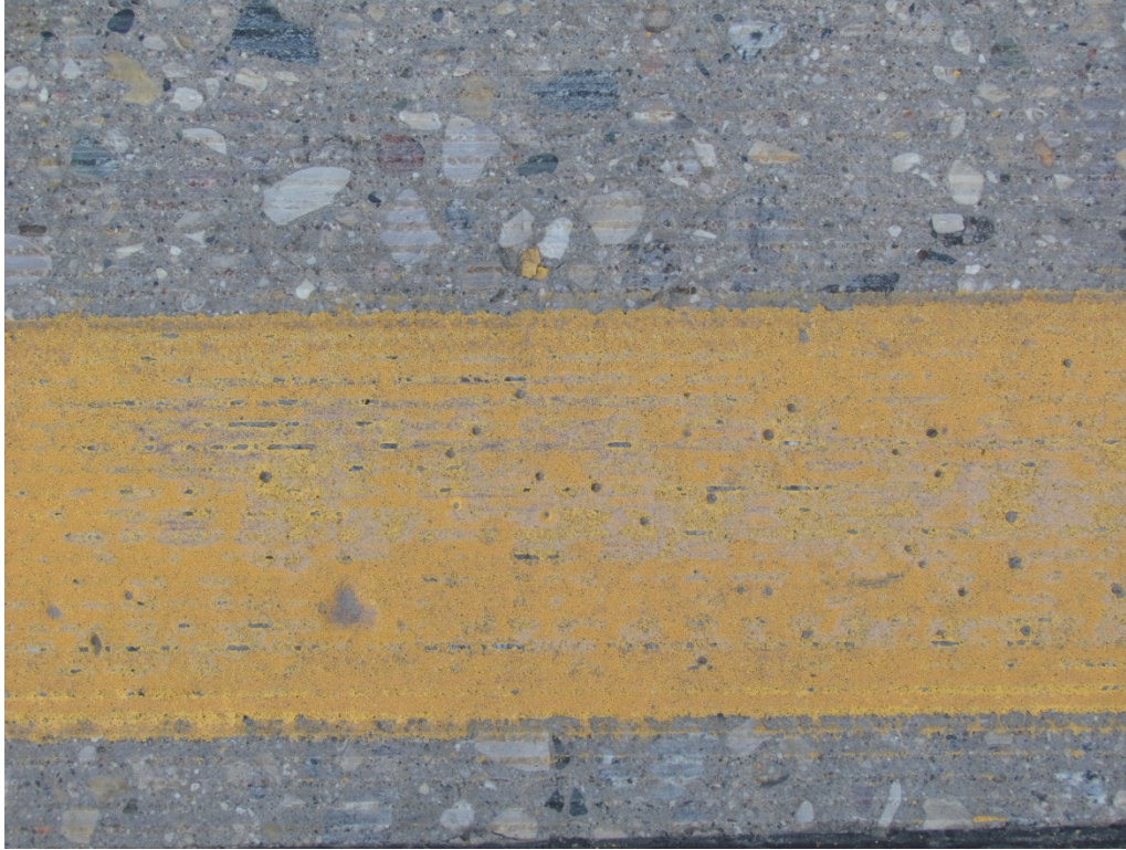
Segment 3A - SB Yellow Surface applied Epoxy with Standard Glass Beads – RP 145
