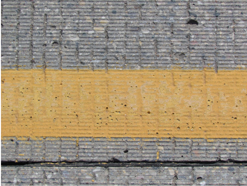
Segment 3A - NB Yellow Surface applied Epoxy with Standard Glass Beads – RP 145
