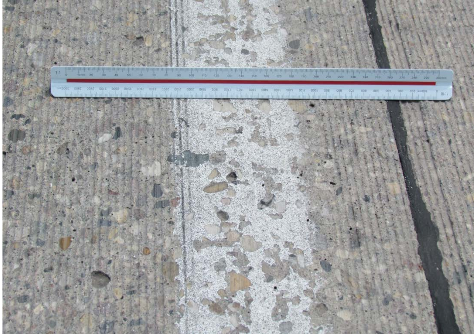
Photo 10: Grooved standard water-based paint with standard glass after 2 winters.
