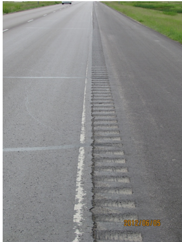
Photo 15: Damaged White Edge-line AWP with AW Elements
