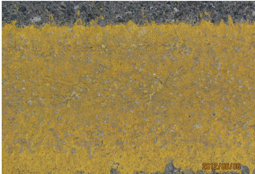
Photo 16: Yellow AWP with Sheared AW Elements
