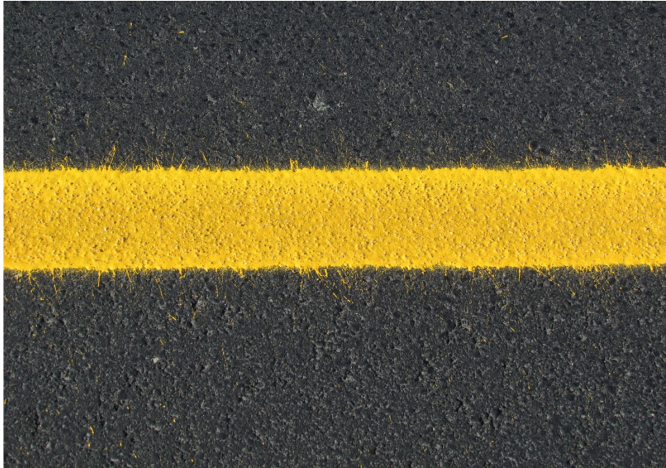
Photo 13: Westbound Yellow AW Paint with AW Elements
