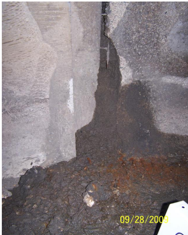
Photo 46: S10 South Haunch
