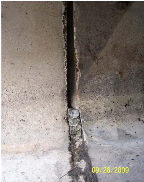
Photo 70: S16 South Haunch
