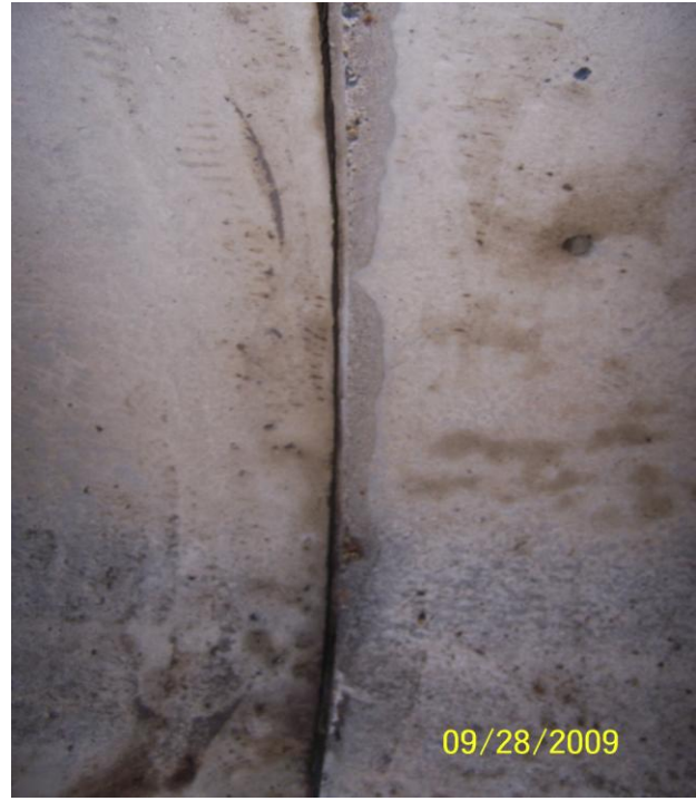
Photo 33: S7 North Haunch
