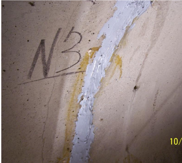
Photo 155: Surface epoxy in 2009
