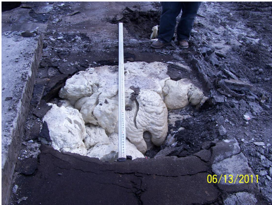
Photo 168: Void 4 directly under the pavement that was \frac{3}{4} full of rigid foam.
