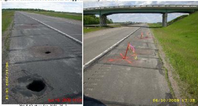
Figure 1: Holes above RCPAs at approximately RP 75.1
