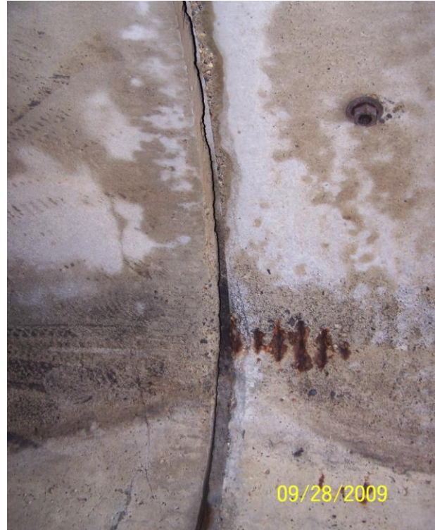
Photo 13: S2 North Haunch
