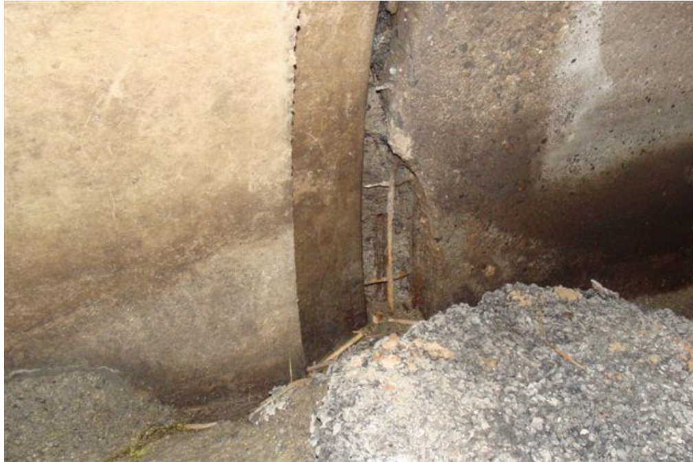
Photo 5: Condition of Joint #10, missing male section of joint, (inventory reference photo 29-002)
