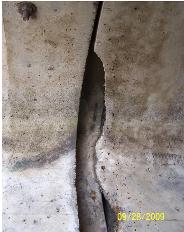
Photo 10: S1 South Haunch
