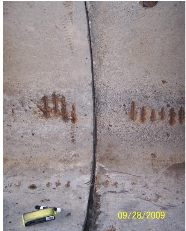
Photo 65: S15 North Haunch
