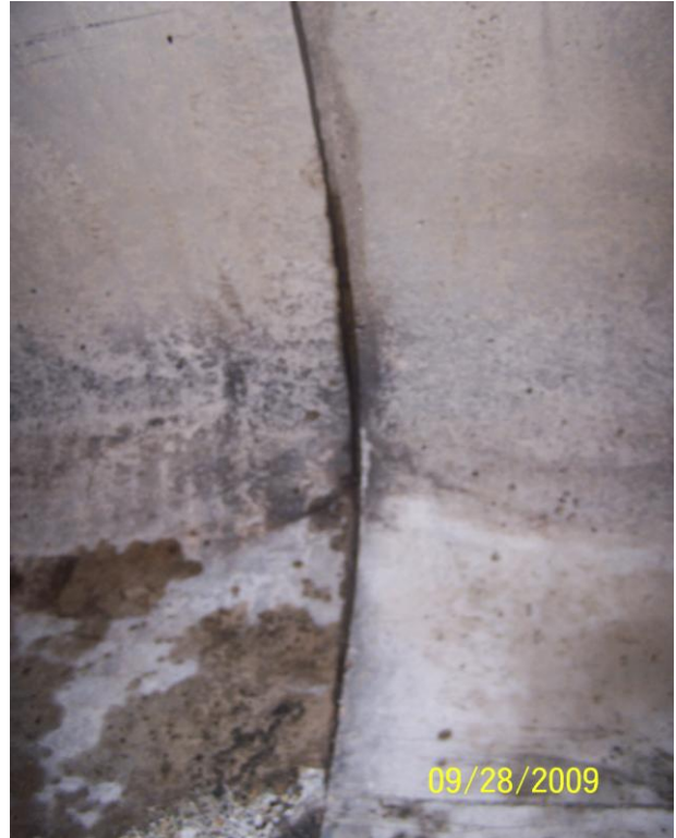
Photo 37: S8 North Haunch
