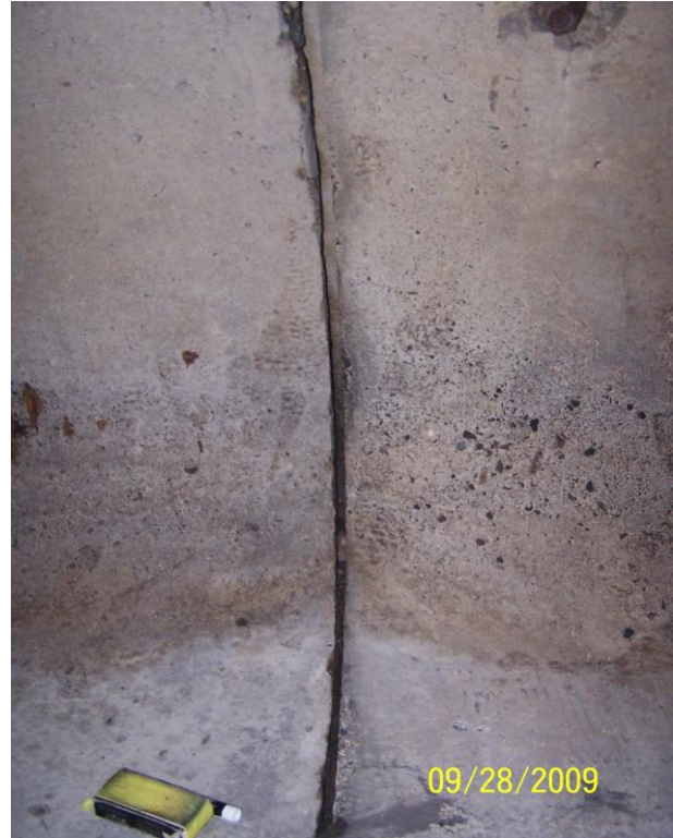
Photo 61: S14 North Haunch
