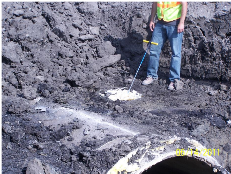
Photo 173: Rigid foam on the exterior of pipe.
