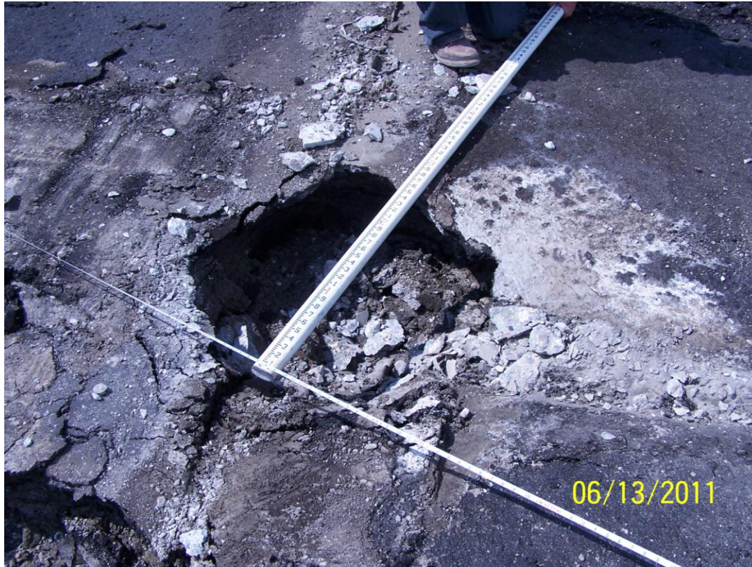
Photo 167: Void 3 directly under pavement surface.
