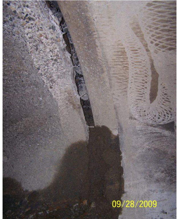
Photo 45: S10 North Haunch
