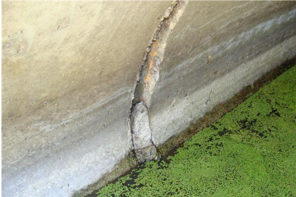
Photo 7: Condition at Joint #14, previous repair (inventory reference photo 29-004)
