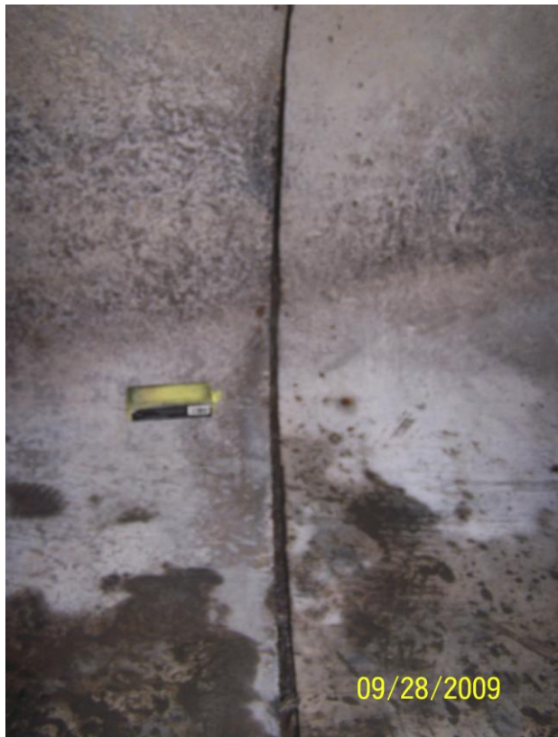
Photo 42: S9 South Haunch
