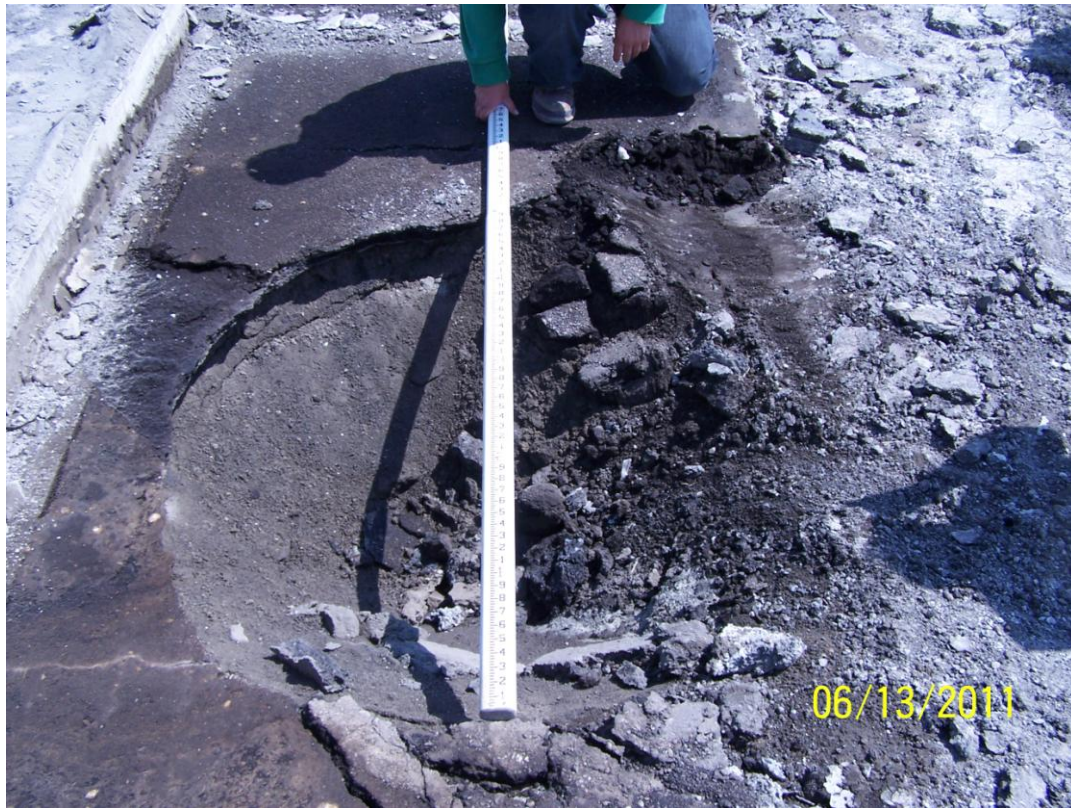
Photo 169: Void 5 directly under pavement surface.
