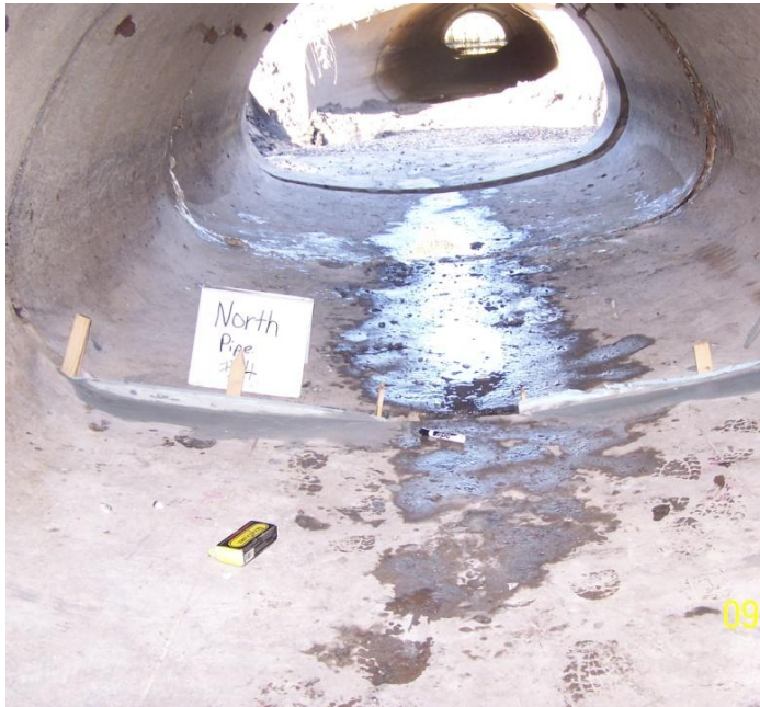
Photo 129: Joint repair in 2009
