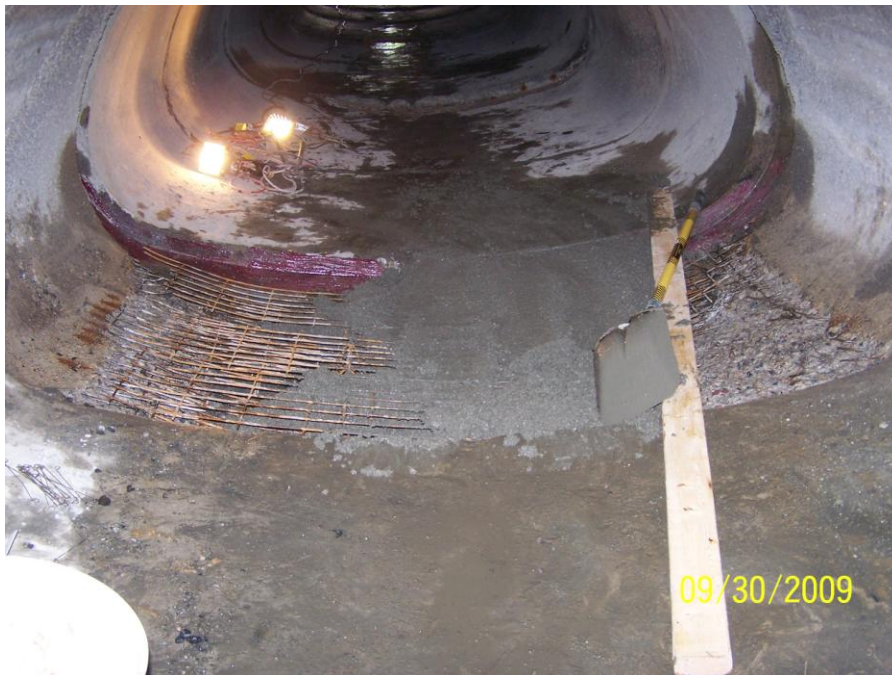
Photo 136: Cretex tied wire mesh to existing steel reinforcement and then filled deteriorated section with concrete
