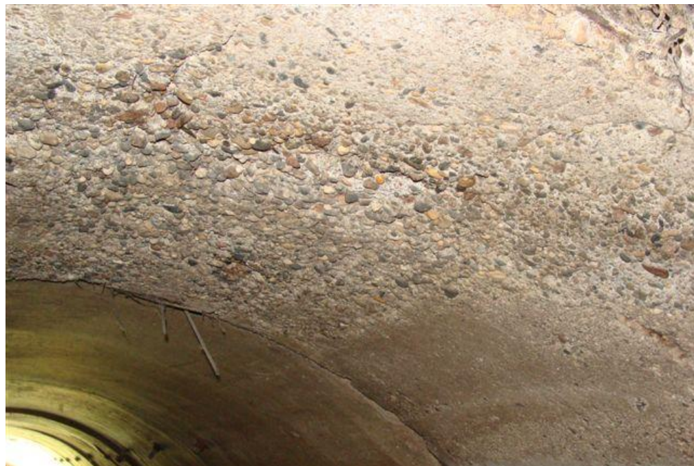
Photo 6: Deteriorated condition of concrete near Joint #10, (inventory reference photo 29-003)
