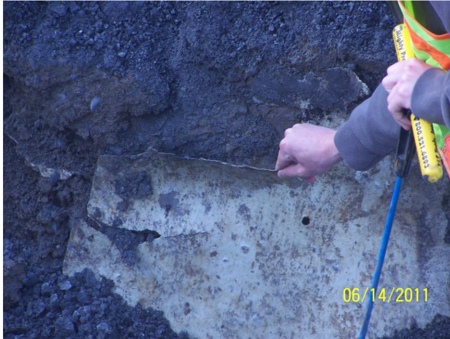
Photo 174: Thin layer of rigid foam found under haunch during excavation.
