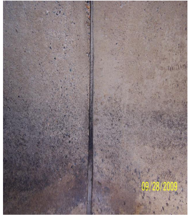
Photo 77: S5 North Haunch
