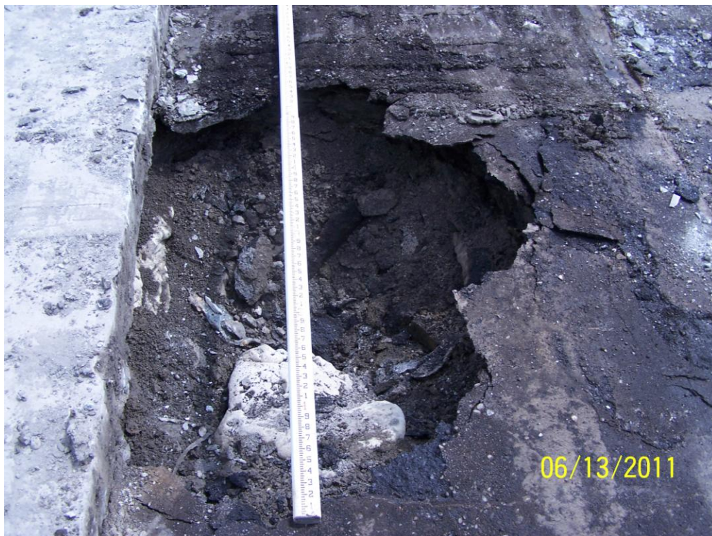
Photo 166: Void 2 top view shows some rigid foam in void.
