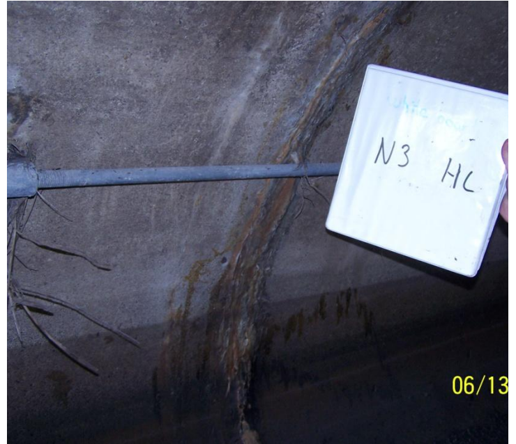
Photo 156: Surface epoxy in 2011
