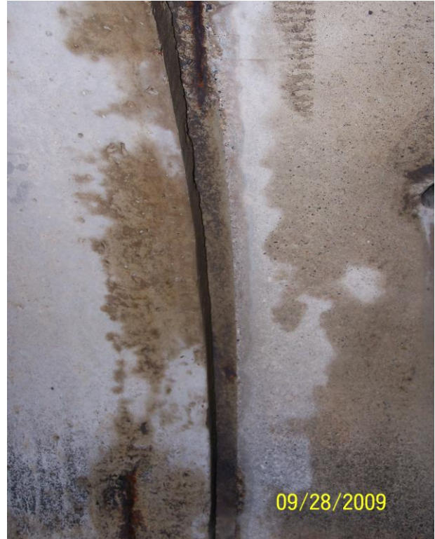
Photo 17: S3 North Haunch
