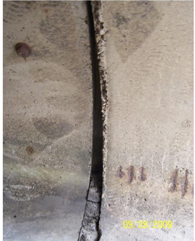
Photo 69: S16 North Haunch
