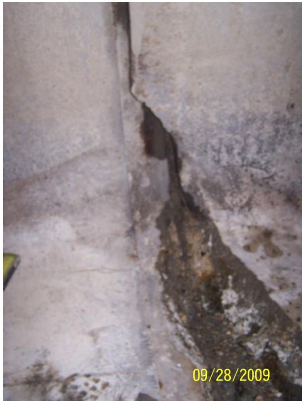
Photo 38: S8 South Haunch
