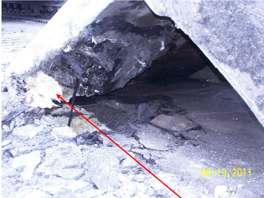
Photo 163: Void 1 that had been filled with rigid foam.
