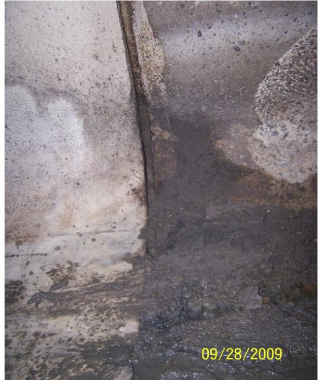
Photo 49: S11 North Haunch
