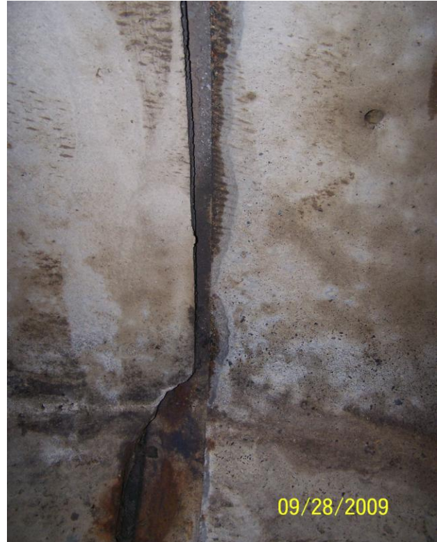
Photo 25: S5 North Haunch
