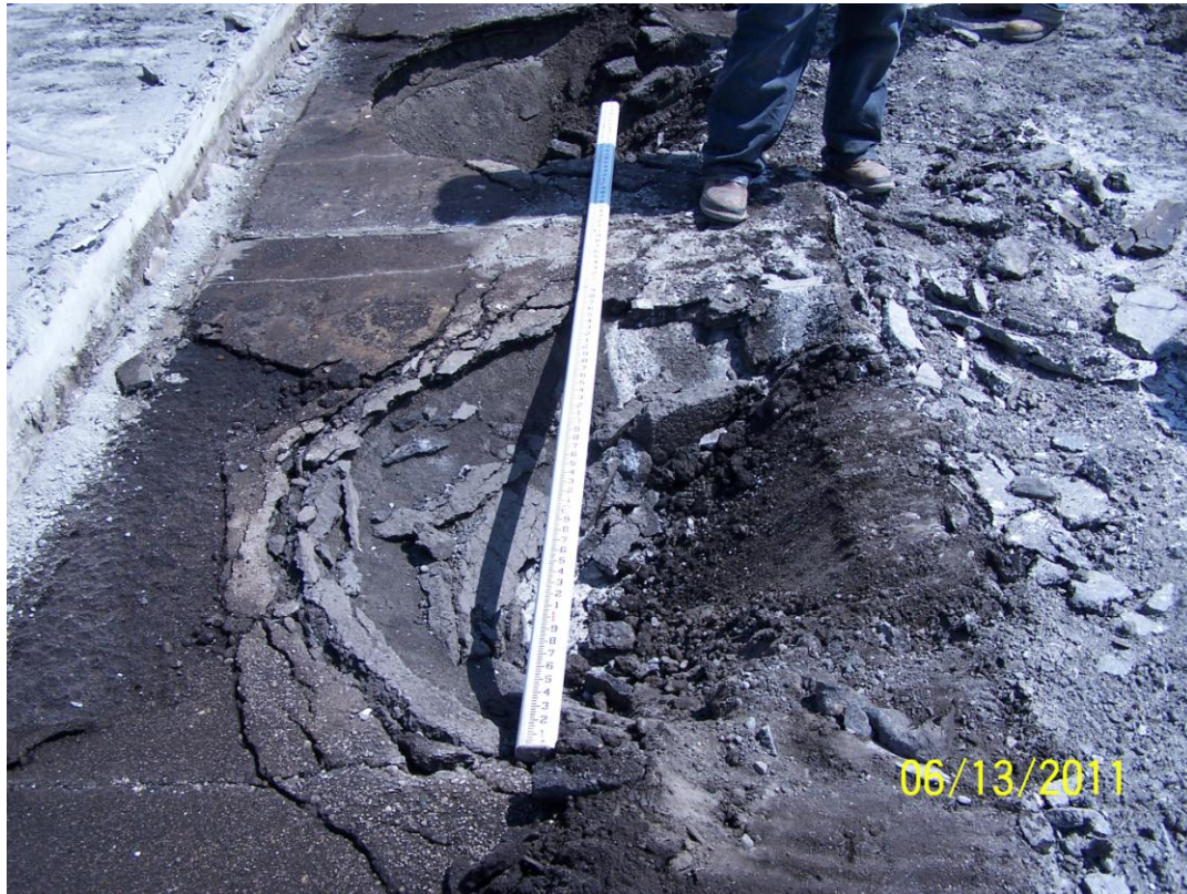
Photo 170: Void 6 directly under pavement surface.
