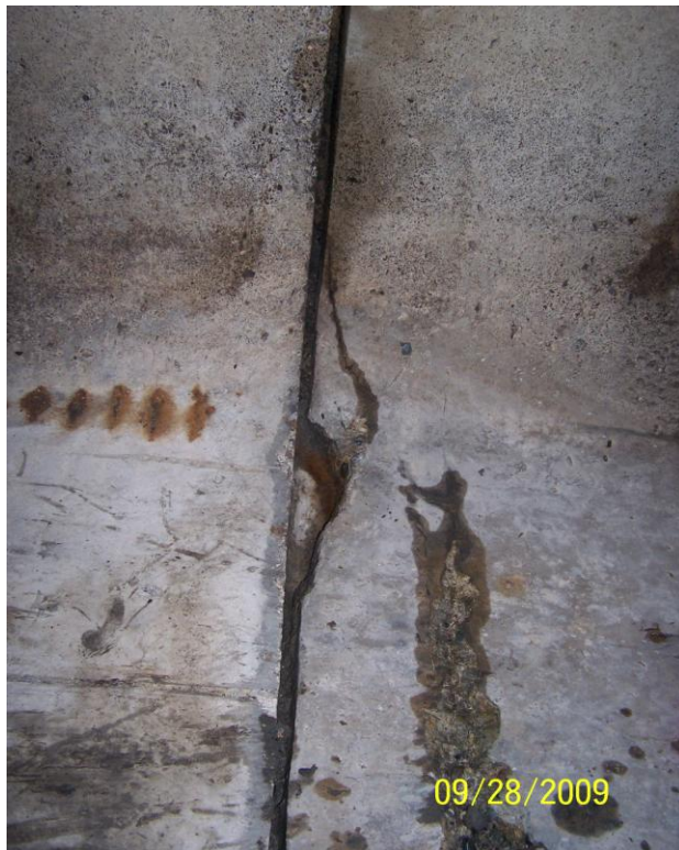
Photo 58: S13 South Haunch
