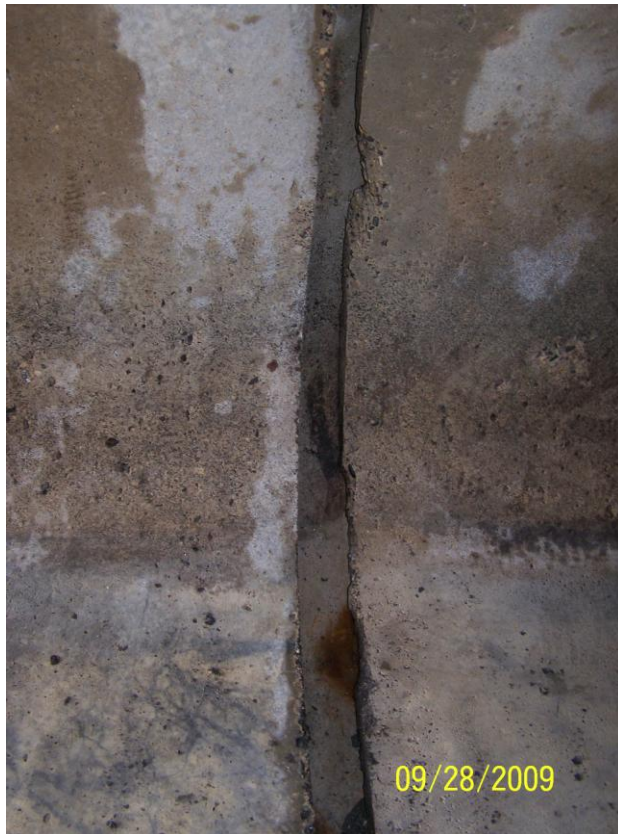
Photo 14: S3 South Haunch
