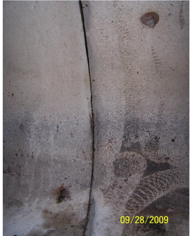
Photo 53: S12 North Haunch
