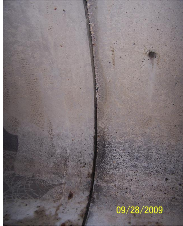
Photo 41: S9 North Haunch
