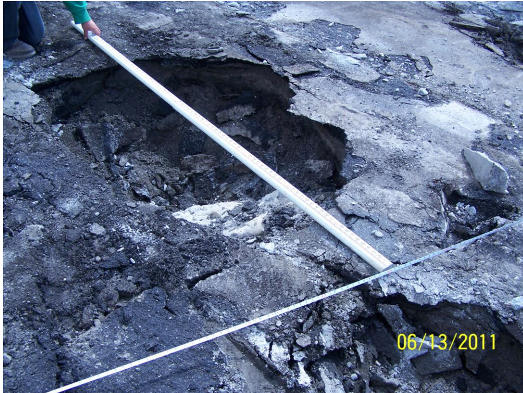
Photo 165: Void 2 directly under the pavement surface.
