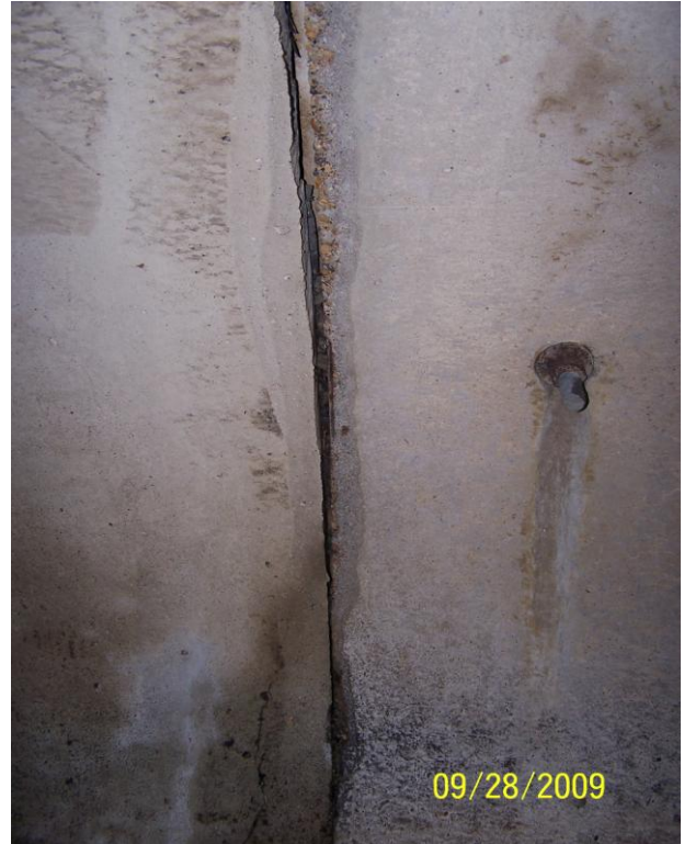
Photo 21: S4 North Haunch
