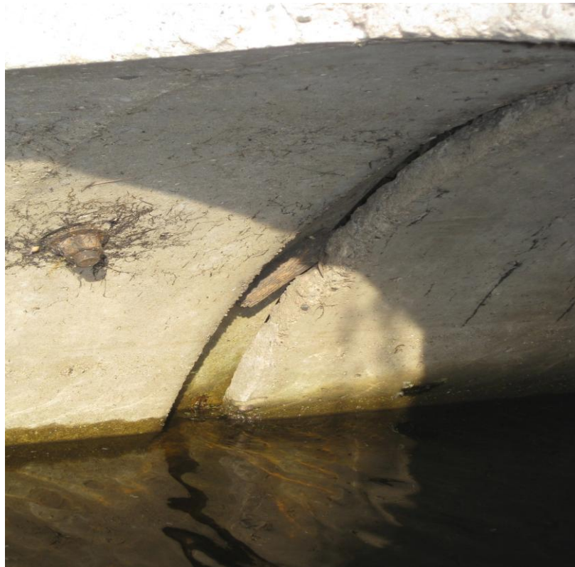
Photo 4: Condition of separated segment
