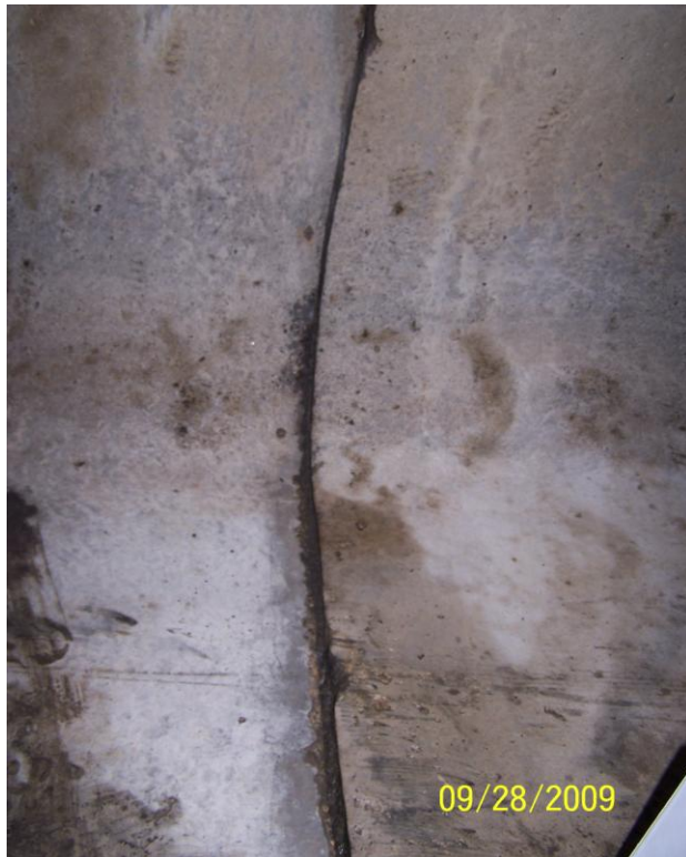
Photo 34: S7 South Haunch
