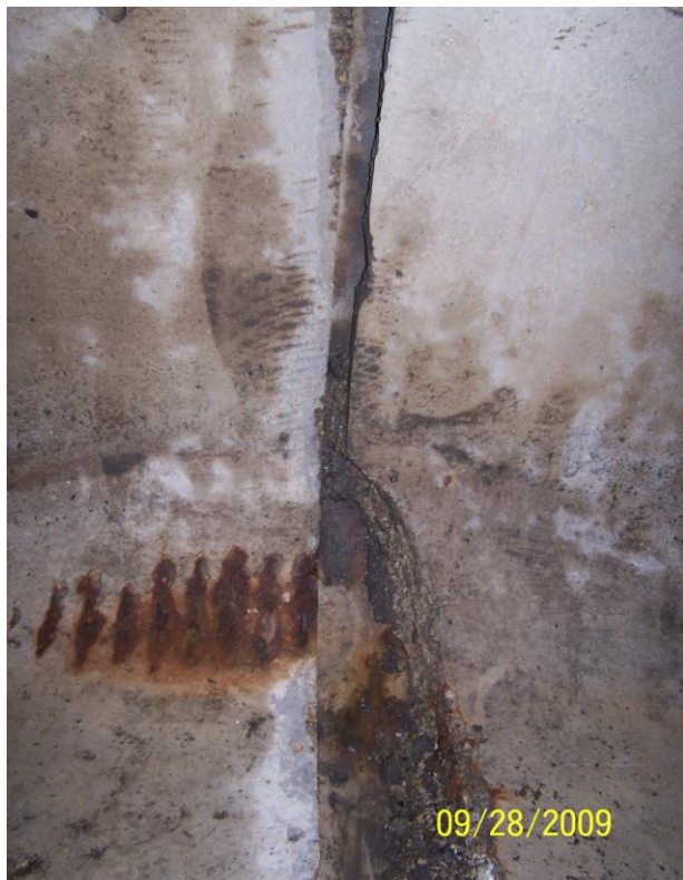
Photo 26: S5 South Haunch
