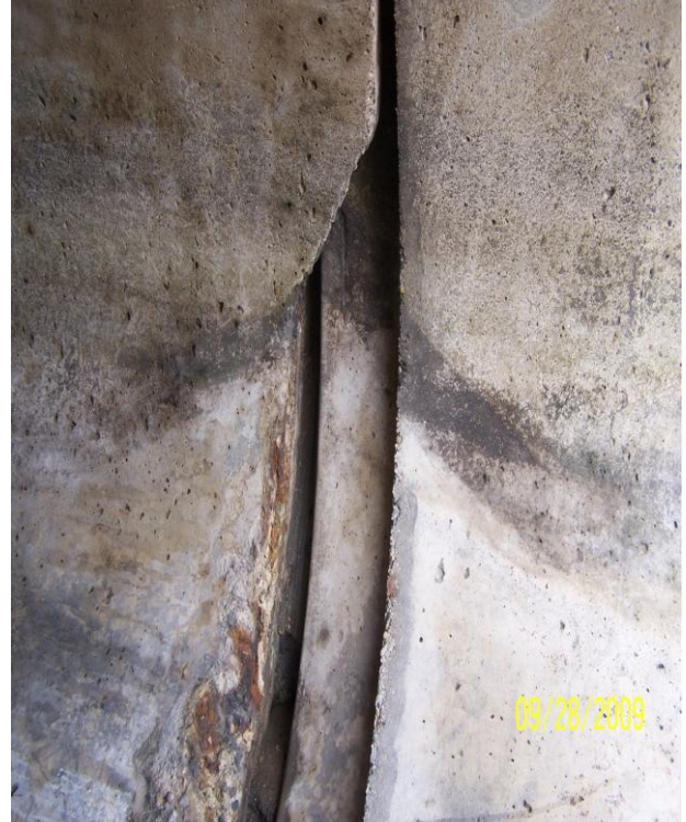
Photo 9: S1 North Haunch
