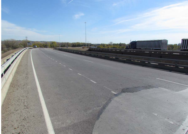
Photo 29: Obliteration Occurring on Part of Installation on the West End of Bridge
