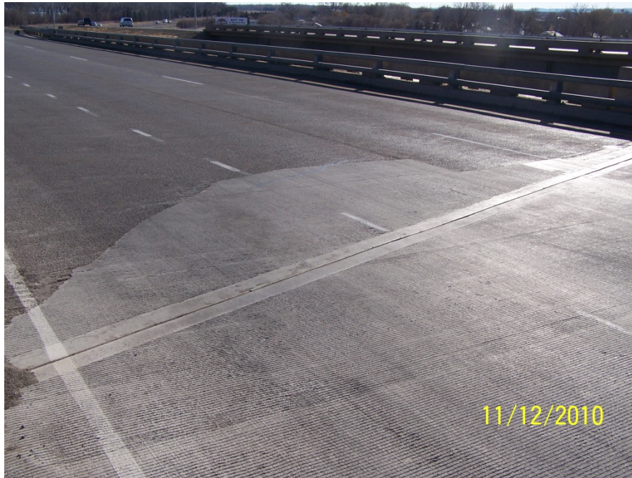
Photo 23: Obliteration Occurred on Part of Installation on the West End
