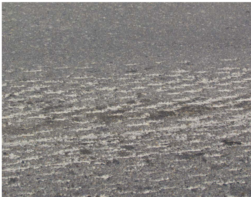
Photo 28: SafeLane™ Bridge Damage
