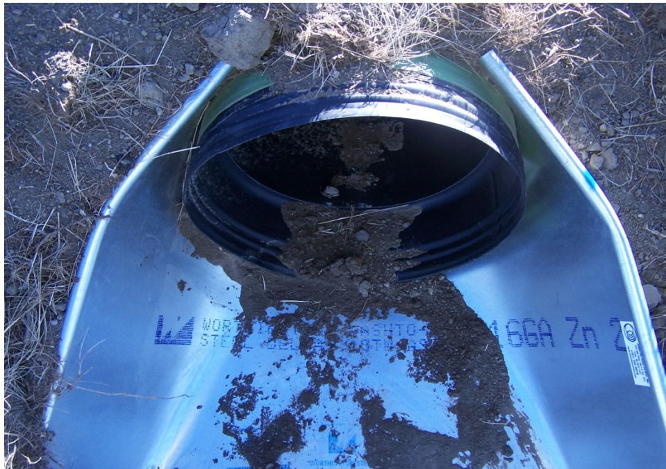
Photo 2: Metal End Section of HDPE pipe.
