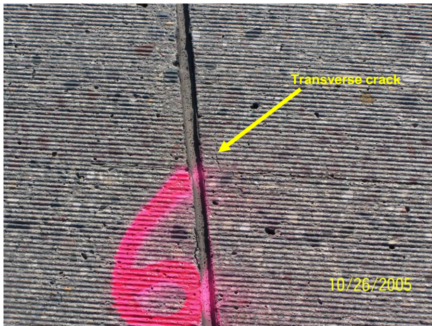
Photo 9 - Transverse crack location is likely the early signs of a coreboard failure.
