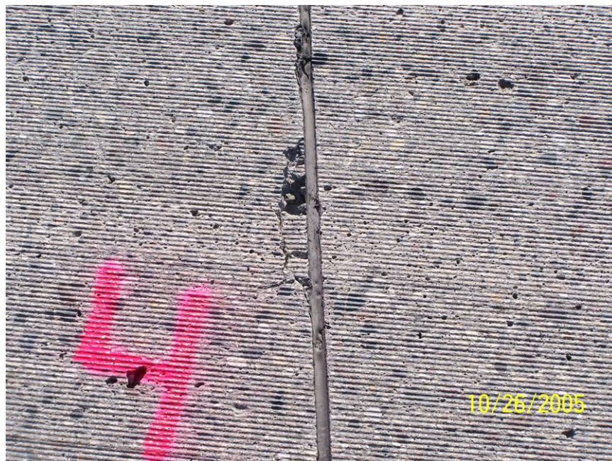
Photo 3 - Spalling at joint and dowel bar slot.
