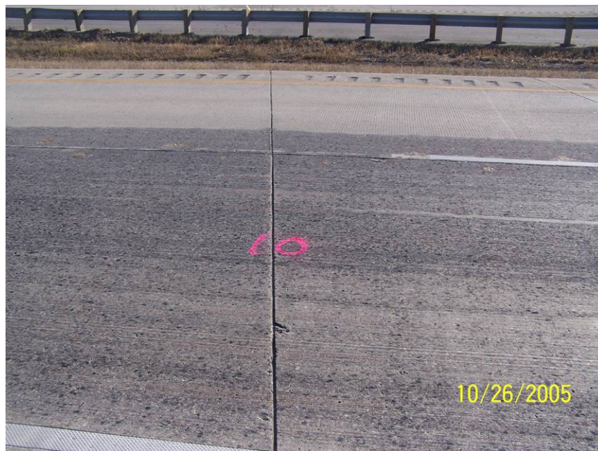
Photo 6 - Typical joint in control section 2 - spall area is in the original PCC pavement.
