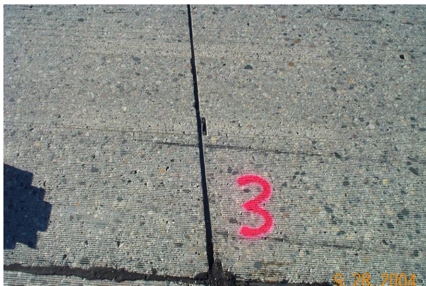
Photo 4 - Coreboard failure in control section 1.
