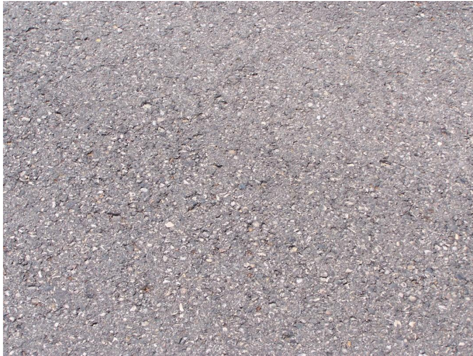
Photo 3 – Area where pneumatic roller tires picked up asphalt
