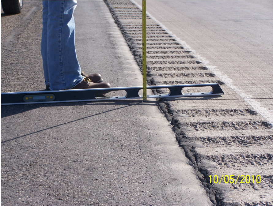
Photo 2 – Settling of the asphalt shoulders in Segment 2.
