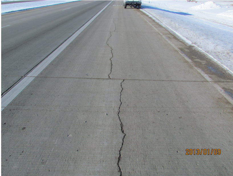
Photo 4 – Longitudinal crack in turning lane in Segment 3.
