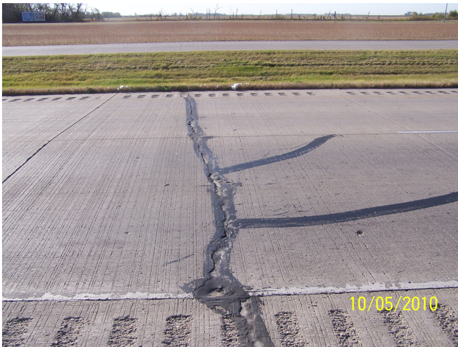
Photo 3: Distress located in Segment 3.
