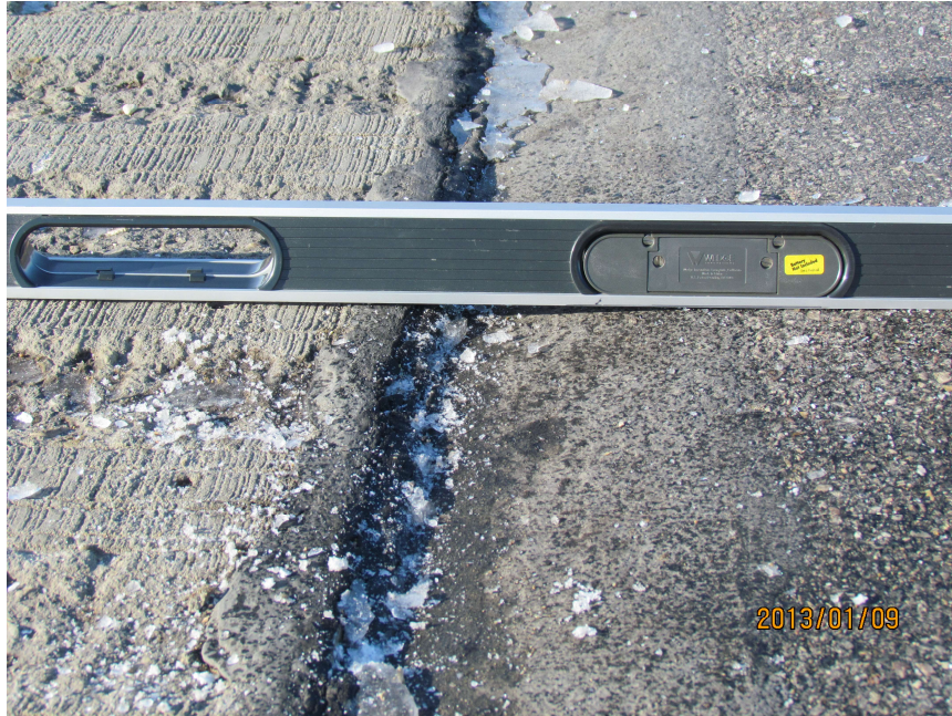
Photo 2 – Settling of the asphalt shoulders in Segment 2
