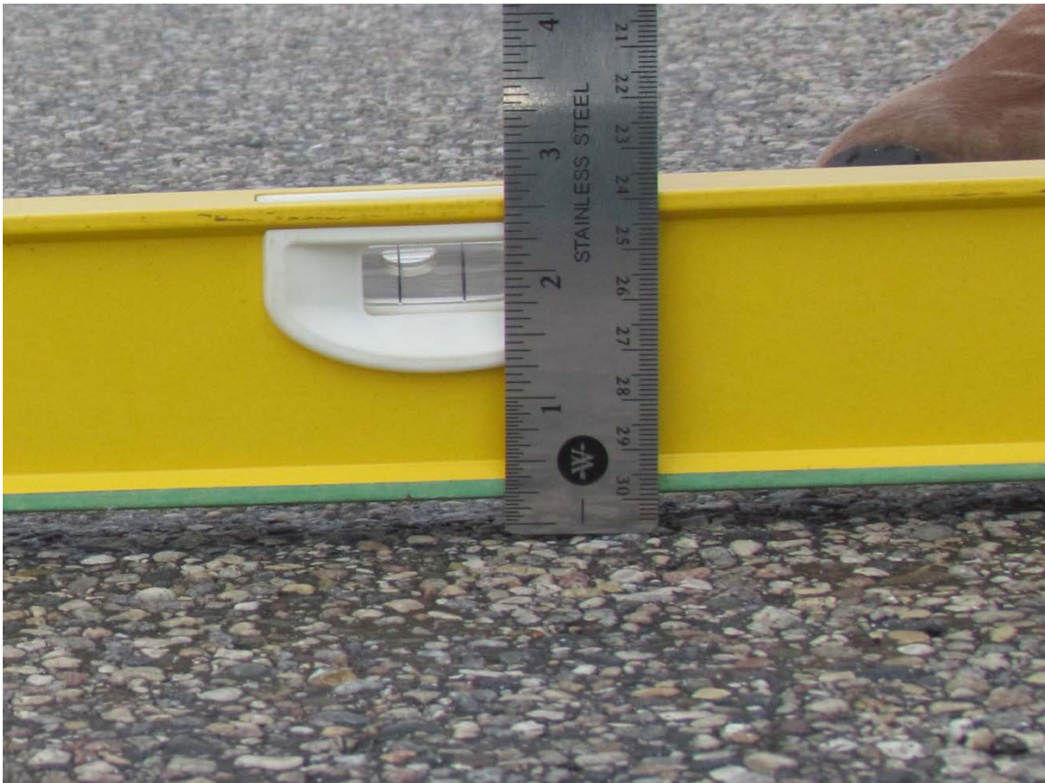
Photo 6, Rutting in Section 3
