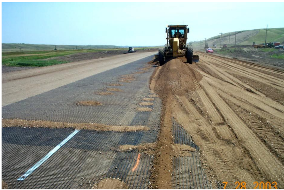
Photo 9 – Spreading base – notice the base material on the geogrid. It keeps the ends down so it stays in place.
