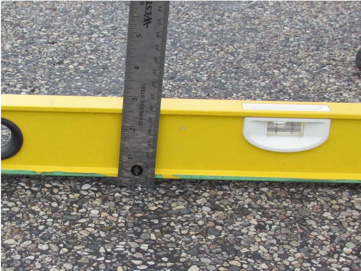
Photo 4, Rutting in Section 1
