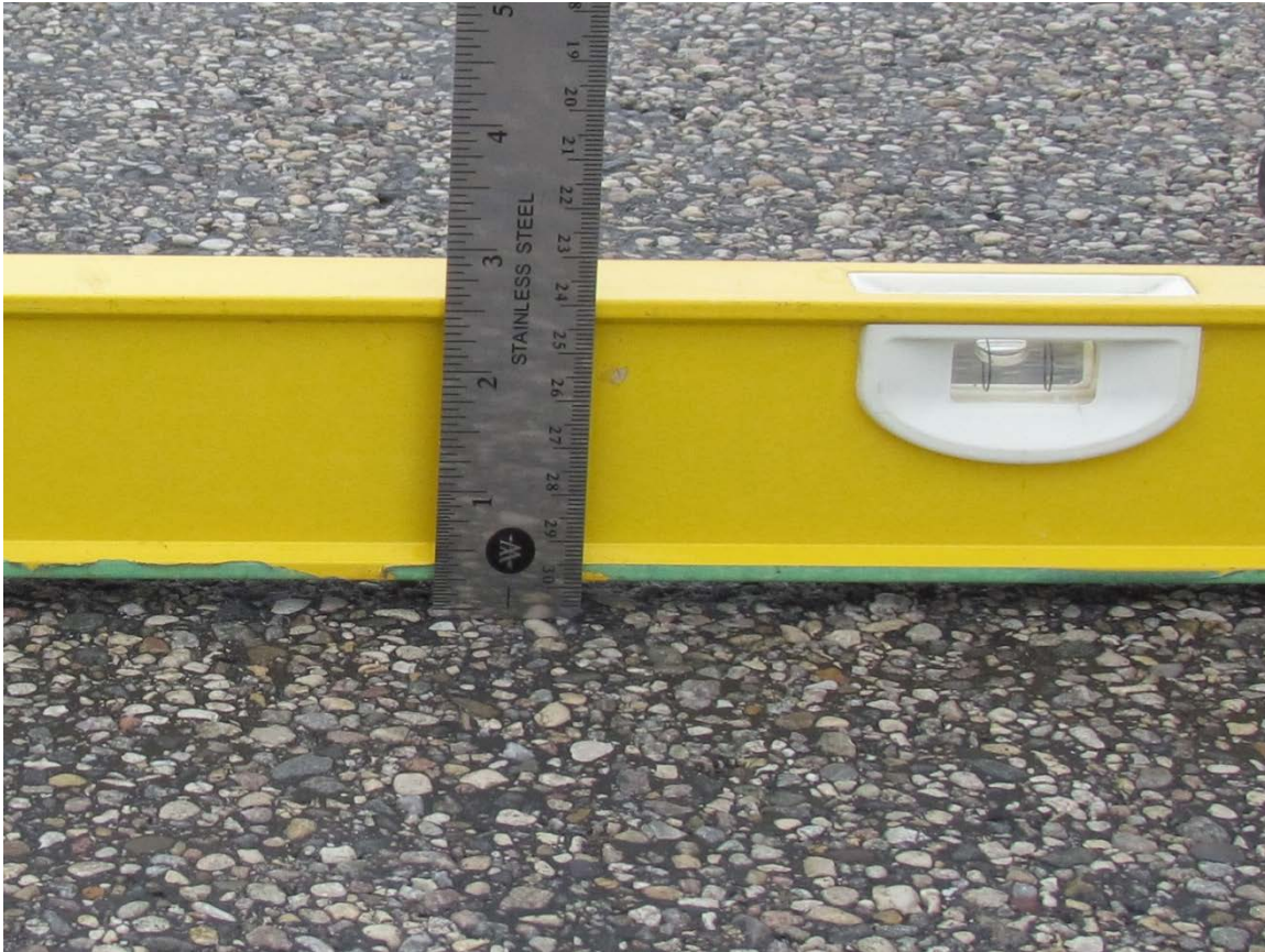
Photo 5, Rutting in Section 2
