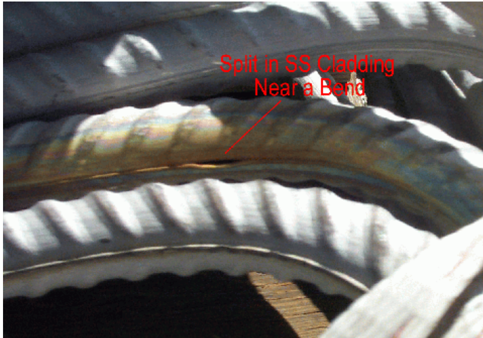
Photo 4. Split in Stainless Steel Cladding near a bend
