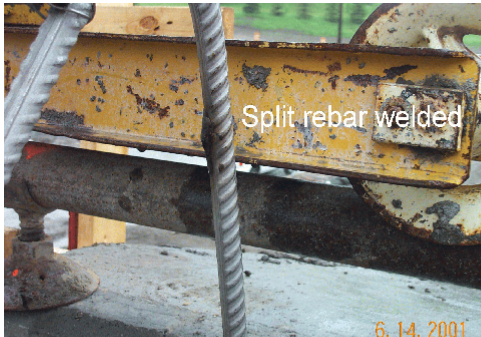
Photo 8. Split rebar welded
