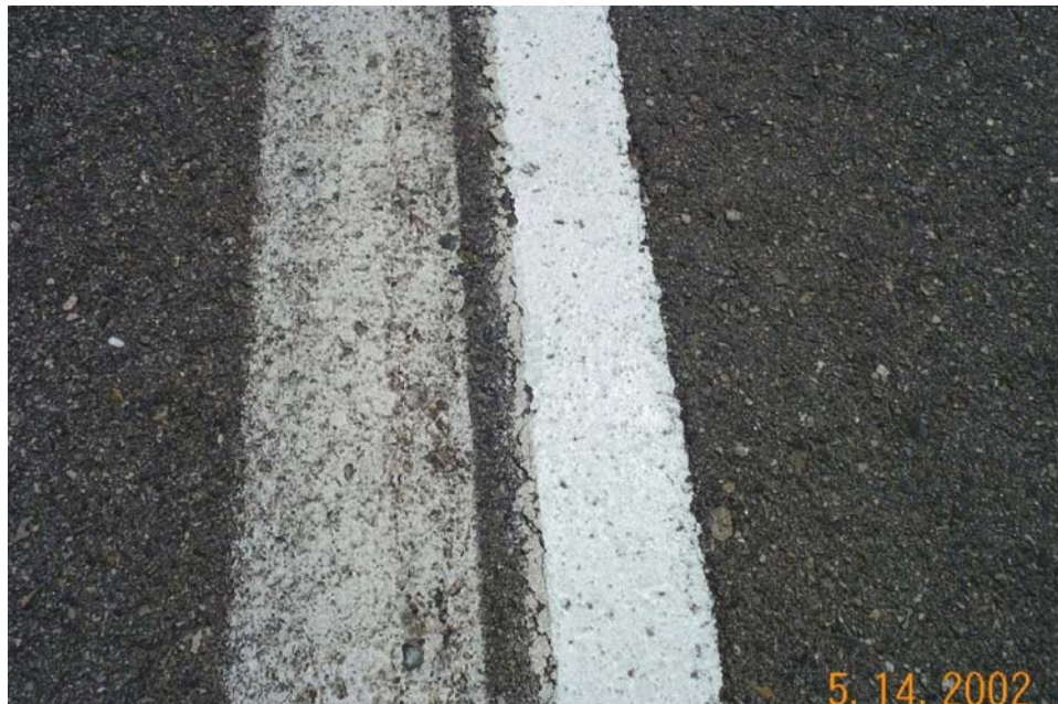
Photo 6 - Left marking is water based paint and the right marking is Series 1200 paint. (Temporary marking placed previous to Series 1200 paint is visible on the left edge of Series 1200 line.)
