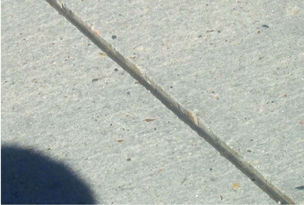
Photo 1 – This is a depressed sealant in a joint on I-94.
