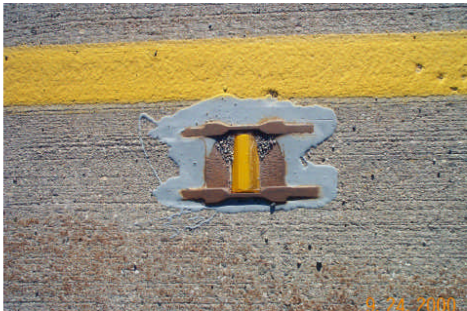
Photo 5 - Debris in recess of marker.
