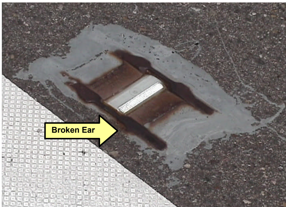
Photo 7 – Marker with oxidized casing and a broken lower right ear.
