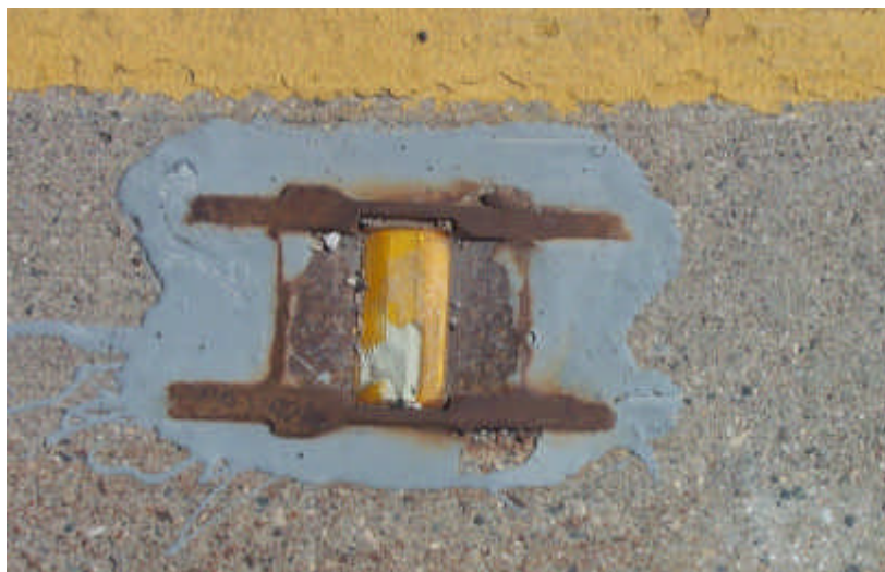
Photo 11 – A marker with a damaged lens at the Interstate 29 ramp installation.
