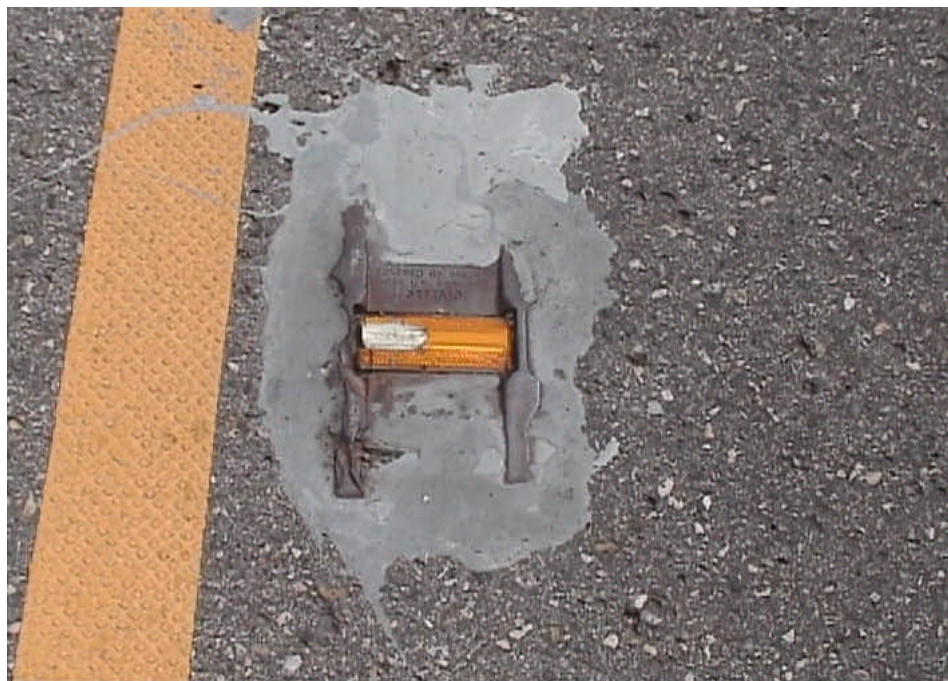
Photo 6 – A damaged marker at the US 52 test section.
