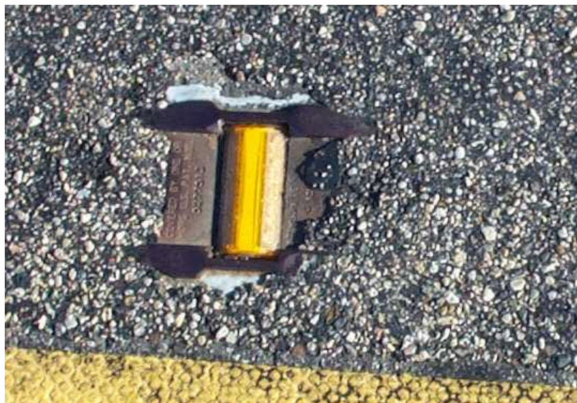
Photo 9 – A raised marker on the US 52 test section after application of a chip seal.
