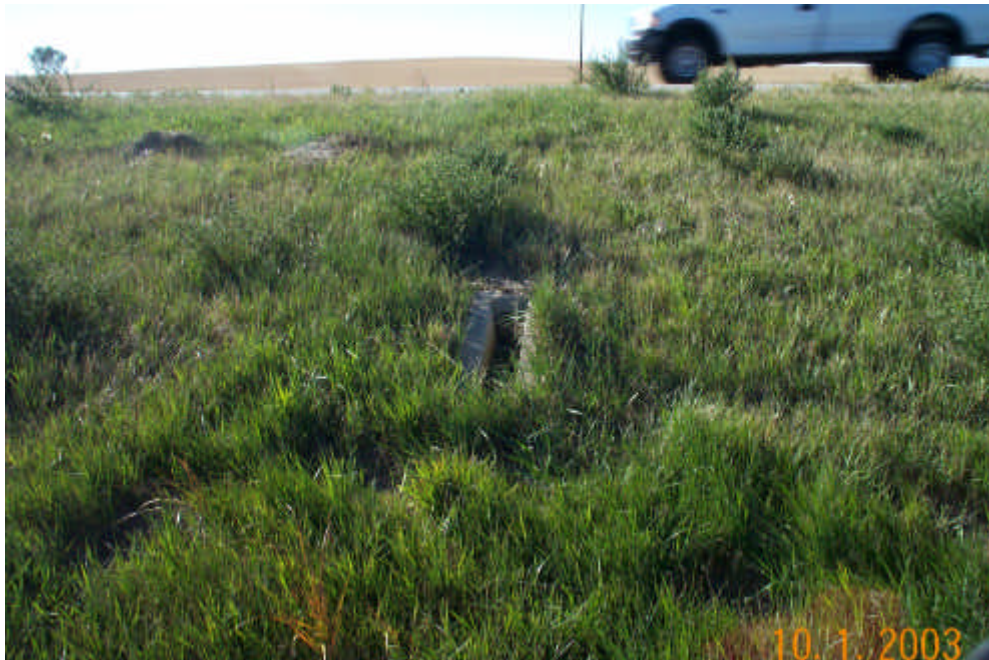
Photo 17 - Aggregate barrier overgrown with vegetation.
