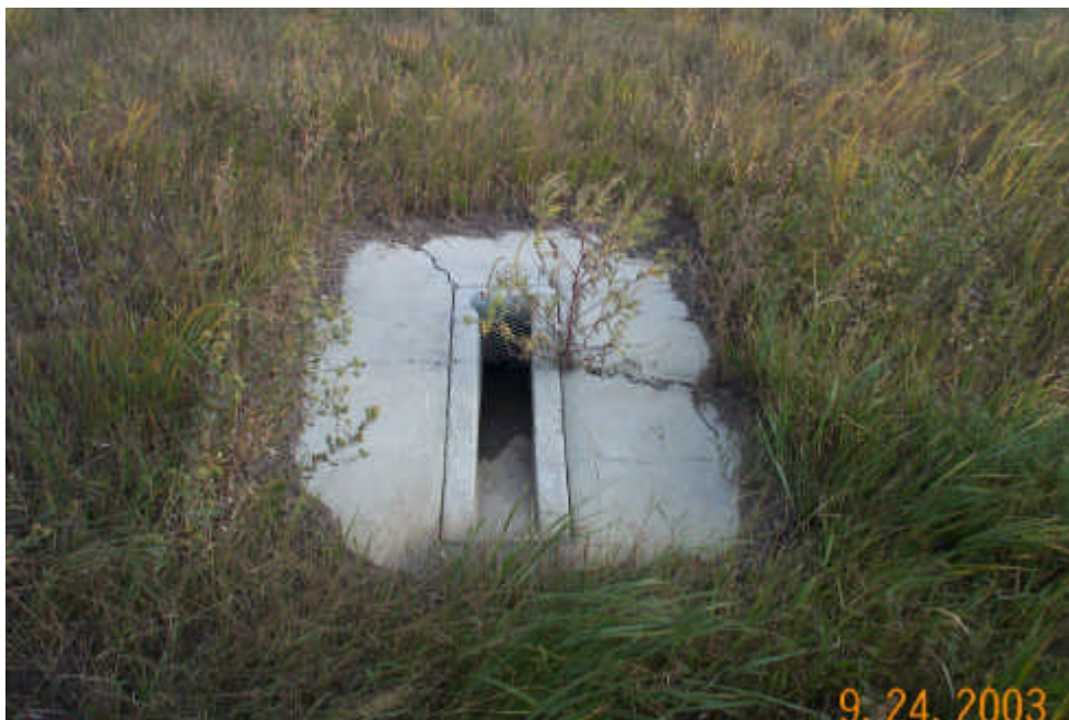
Photo 18 - Cracked concrete barrier.
