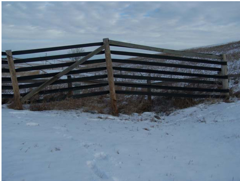
Photo 14 – A fence with tilted posts in wet soil at Site 1.
