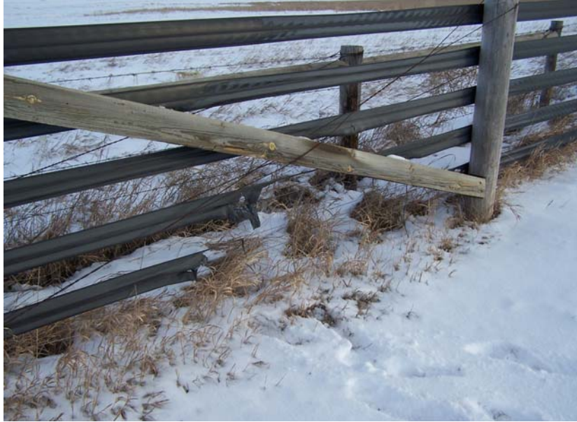
Photo 13 – Damage to polymer straps caused by a grass fire. Note that the internal steel wires remained intact.
