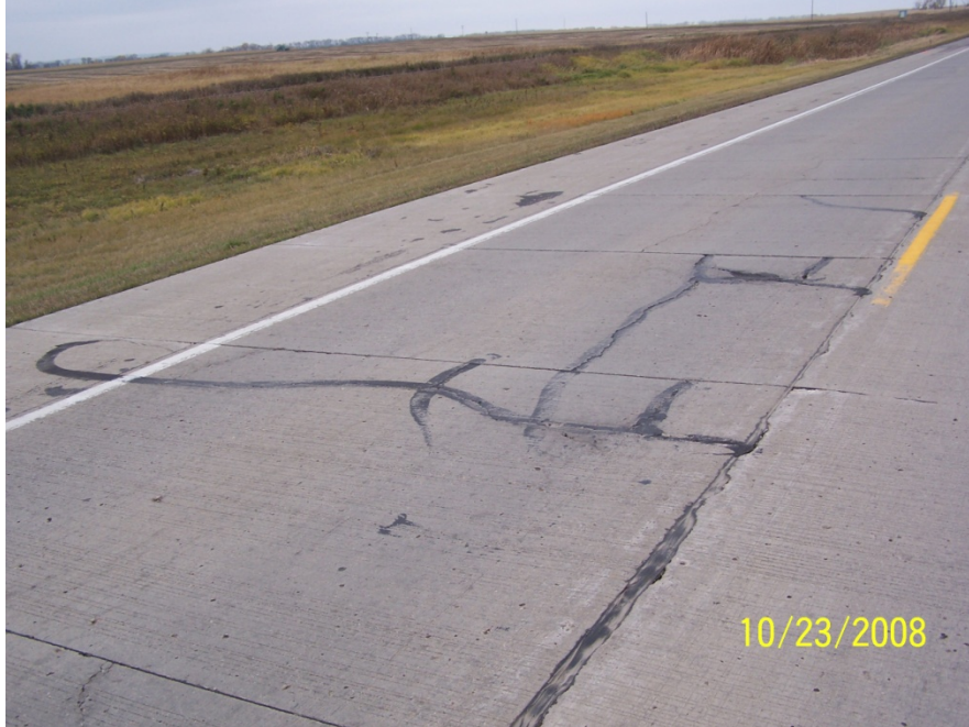
Photo 9 - Longitudinal and Transverse cracks in test section 1
