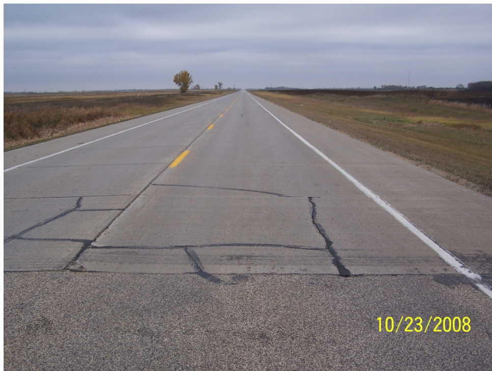
Photo 15 – Block crack in test section 3 looking North on 10/23/08
