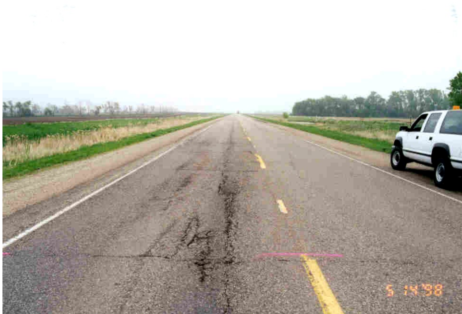
Photo 1 - Overview of distressed areas on a segment of US 52.
