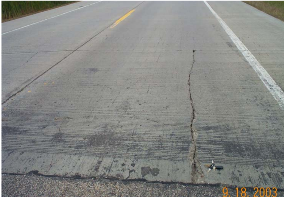
Photo 14 - Longitudinal crack in test section 3 looking north on 9/18/03.
