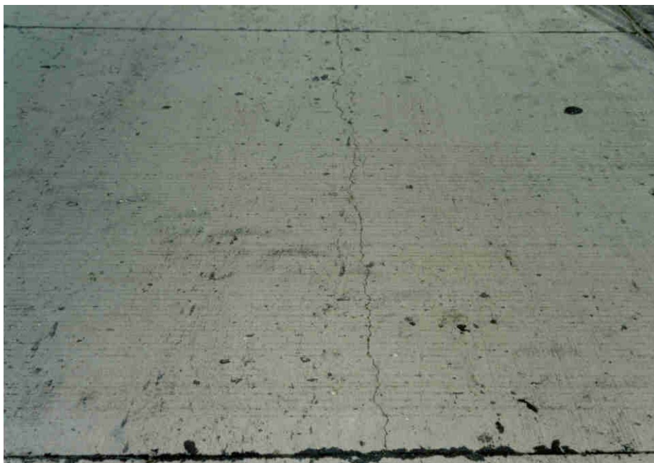
Photo 8 - Longitudinal crack in test section 1 after construction.
