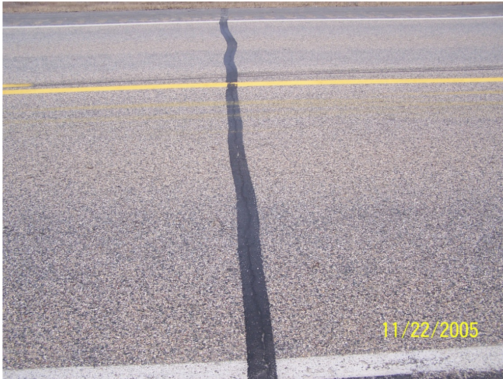
Photo 17 - Transverse Crack in Asphalt Control Section
