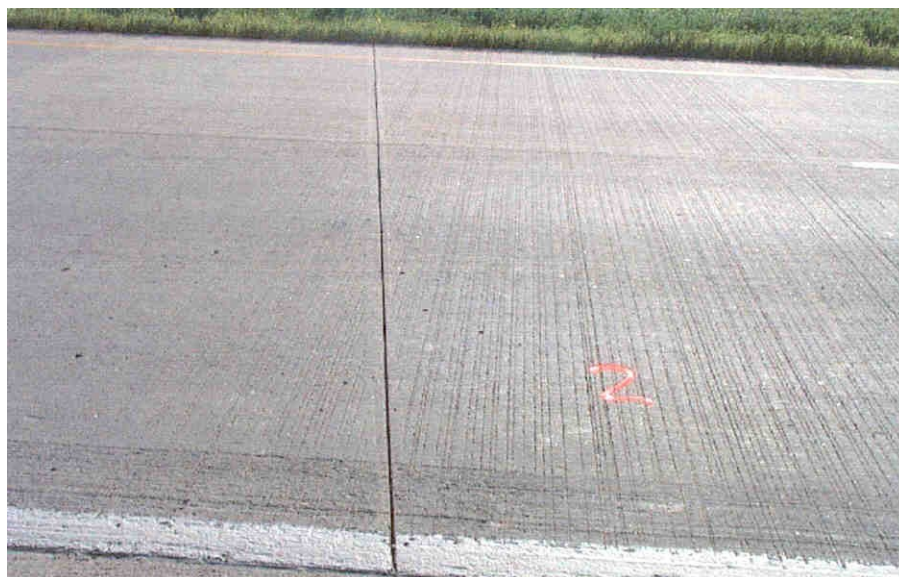
Photo 10 - Typical transverse joint in Test Section 2 and pop-outs.
