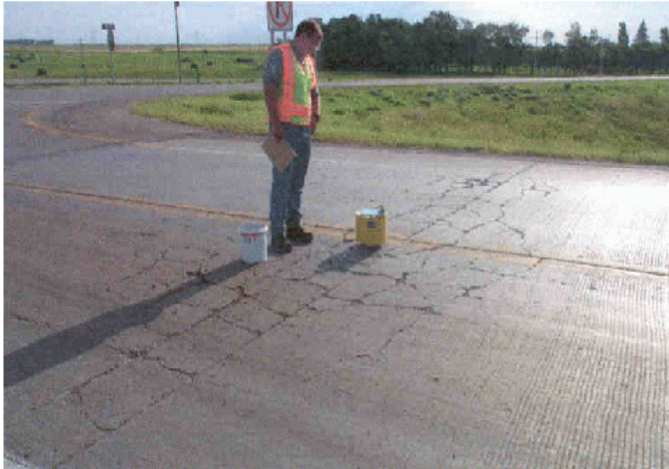
Photo 7. Map cracking occurring at the first joint on the north side of the project.
