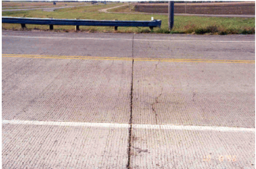
Photo 8. Shows the 1 st joint on the north side of the project in 1998.
