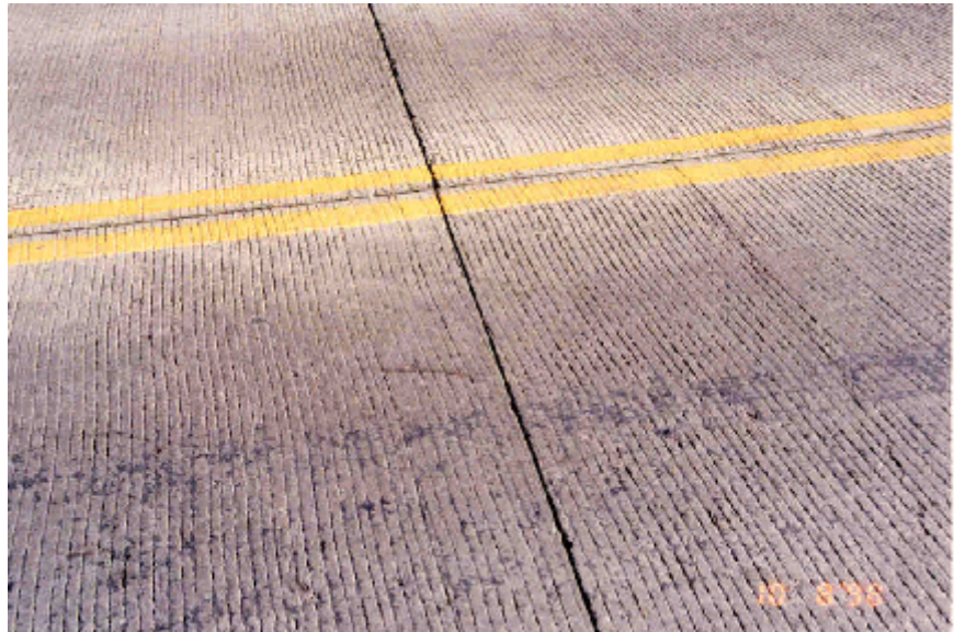
Photo 10. Shows the 2nd joint on the north side of the project in 1998.
