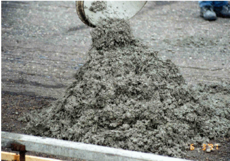
Photo 3. A view of the polyolefin fiber PCC as it is discharged from the mixing truck.
