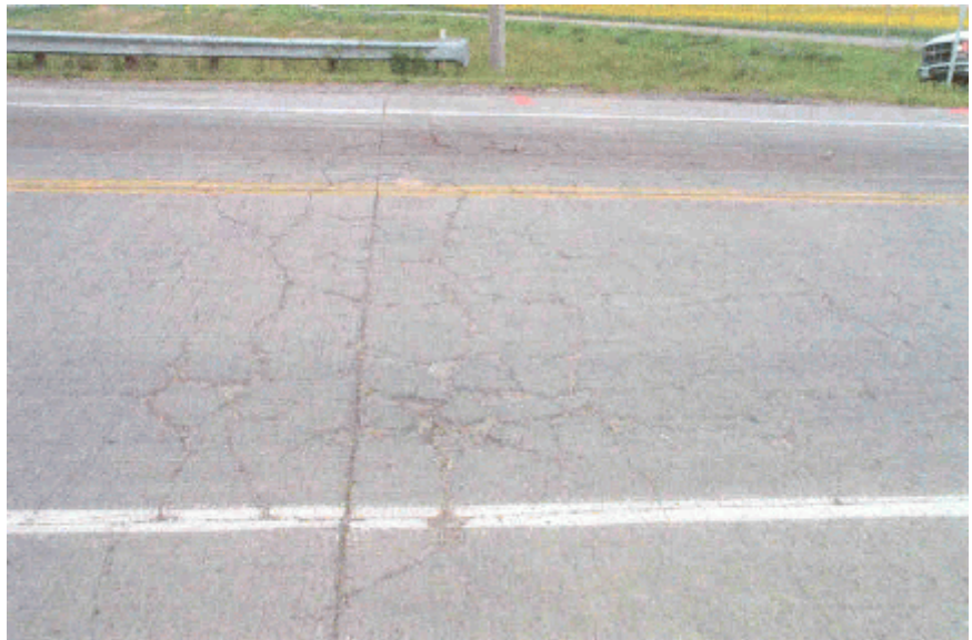
Photo 9. Shows the same joint as in photo 8, but in 2001.
