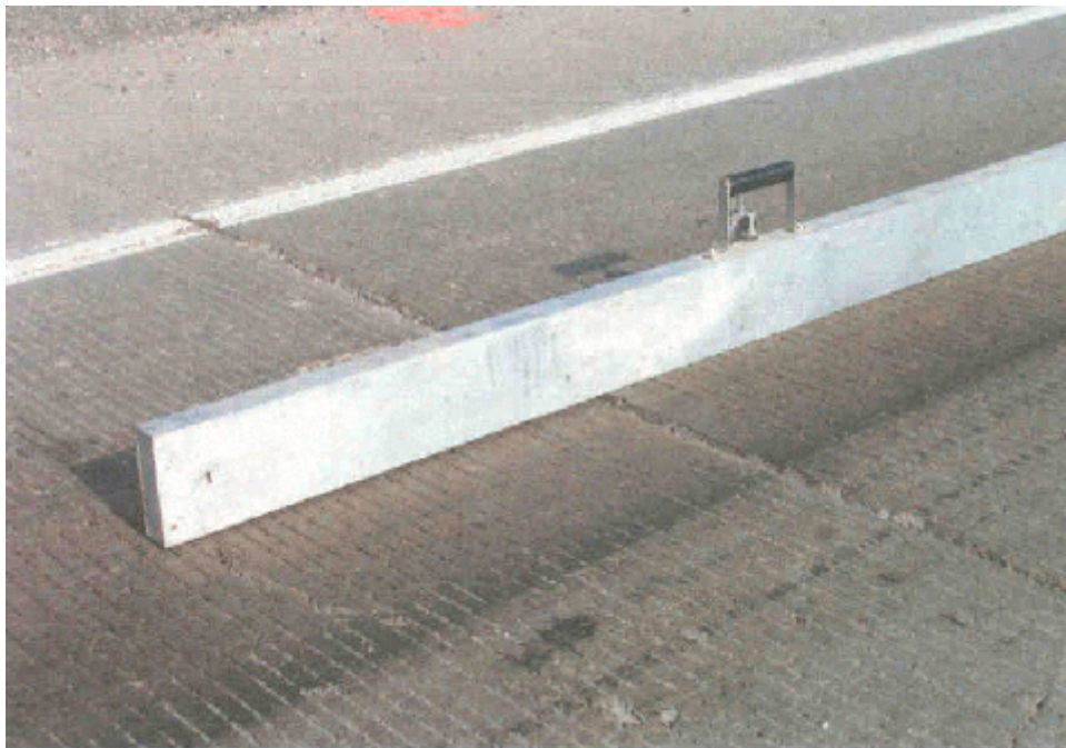
Photo 12. Faulting that has occurred in the SB lane
