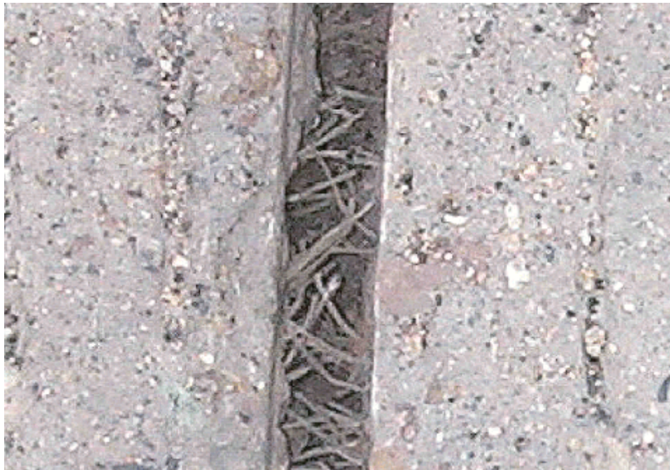
Photo 13. Fibers have broken after joint widening has occurred
