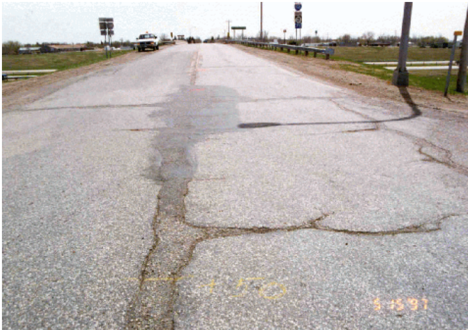
Photo 2. An overview of the existing roadway, prior to milling, where the whitetopping section is now located (looking south).
