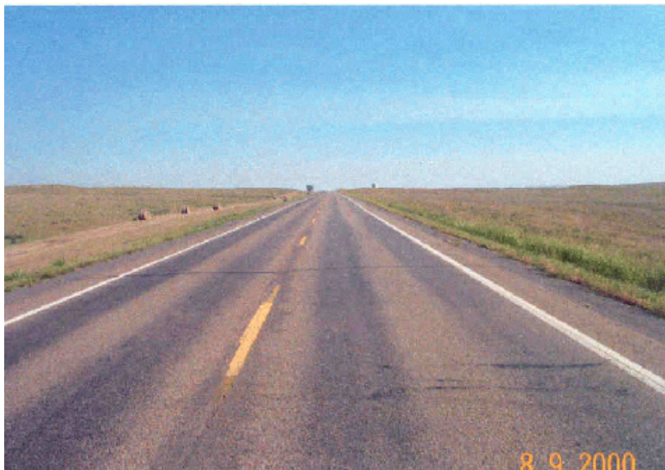
Photo 11 Bleeding in wheel paths
