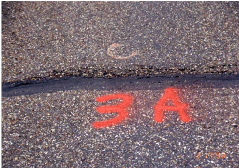
Photo 8 Depressed and multiple cracking--Crafcoc 221 section
