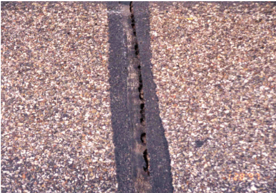
Photo 6 Crafco 221-adhesion failure
