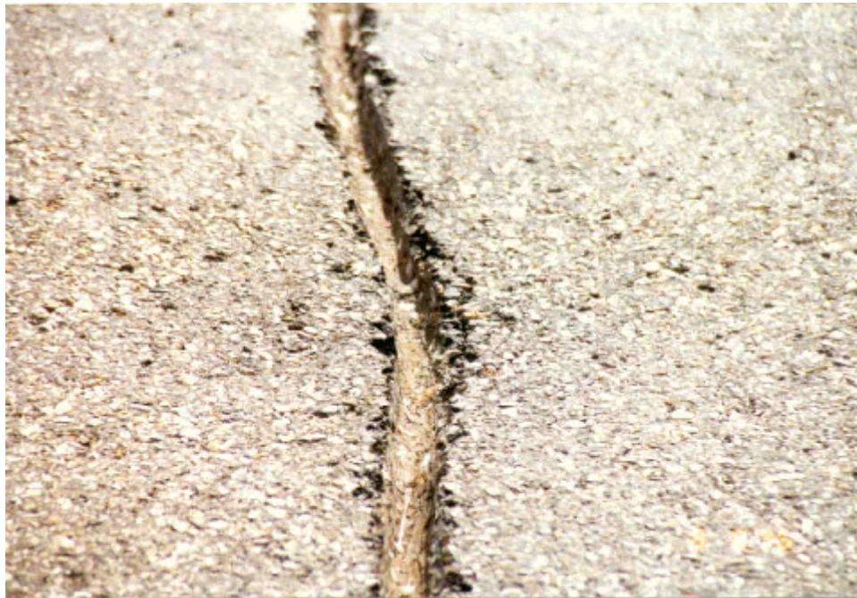
Photo 1 Poor reservoir---worn cutting wheels on router.
