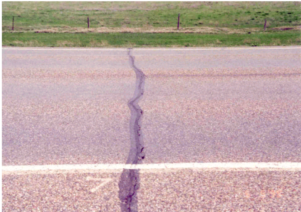
Photo 10 Crafcro 231 section–Same crack as Photo 9 except taken on May 5, 1999 You do not see as much failure–even though it is there
