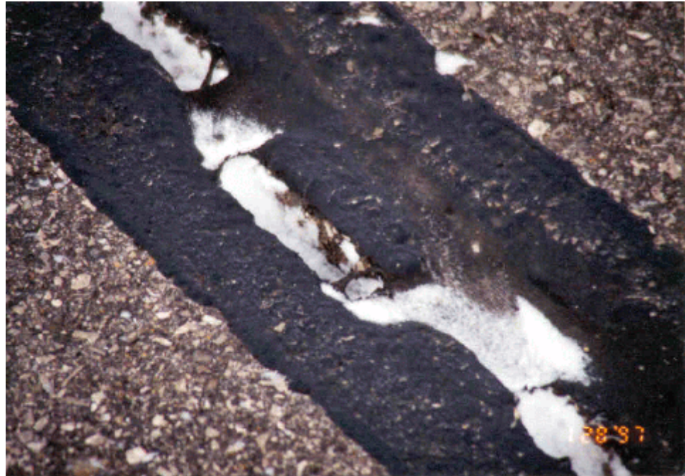
Photo 3 Crafcro 231–failure–routing missed crack (winter 96/97)
