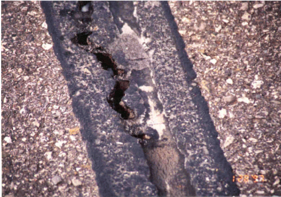
Photo 5 Crafco-failure-routing missed crack (winter 96/97)
