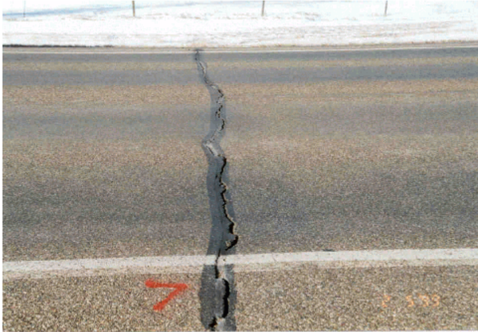
Photo 9 Crafcro 231 section – February 1999 crack severity level
