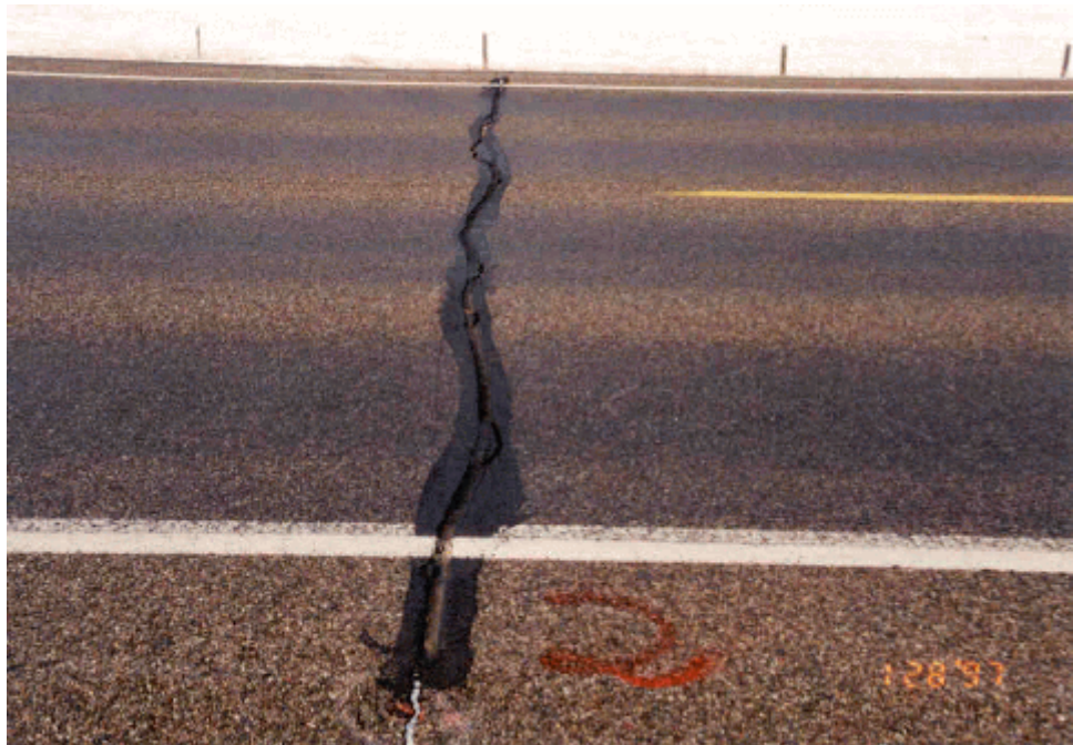
Photo 4 Crafcro 230–failure–routing missed crack (winter 96/97)
