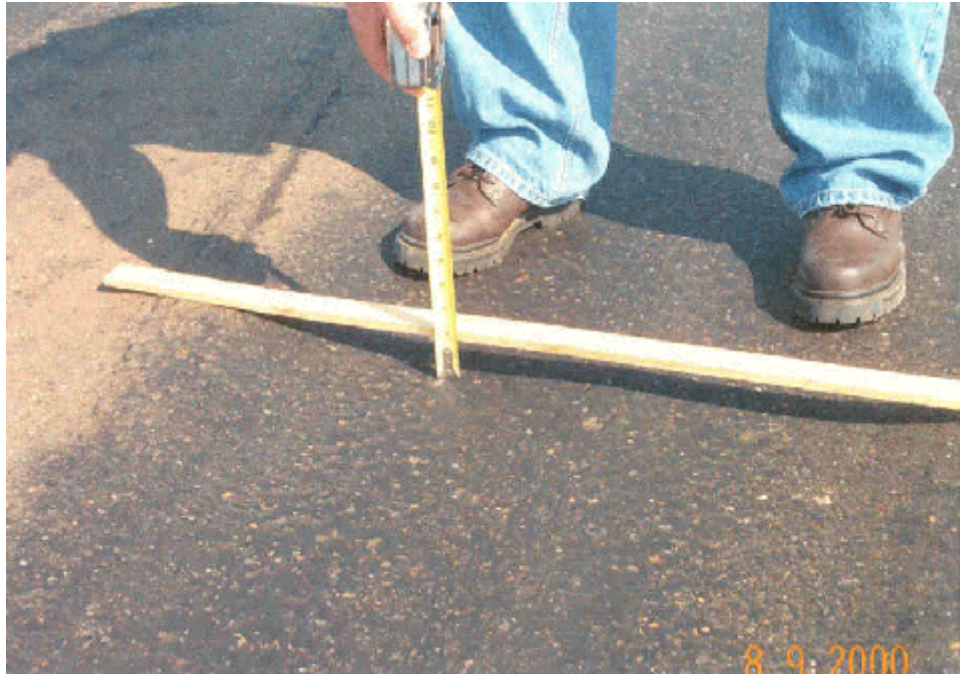
Photo 12 Rutting in inside wheel path – SB
