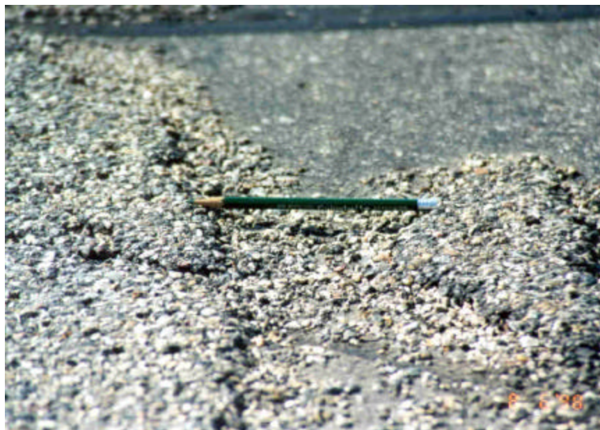
Photo 21 - Distress area shown in the two previous photos.
