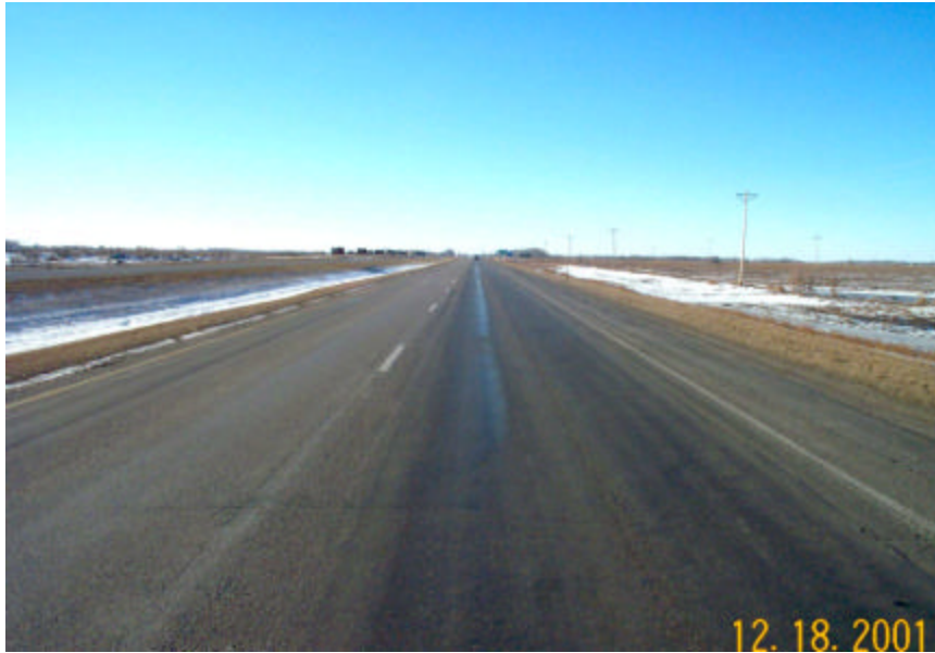
Photo 31 - Bleeding on Highway 2. City of Grand Forks to the Grand Forks Air Force Base.
