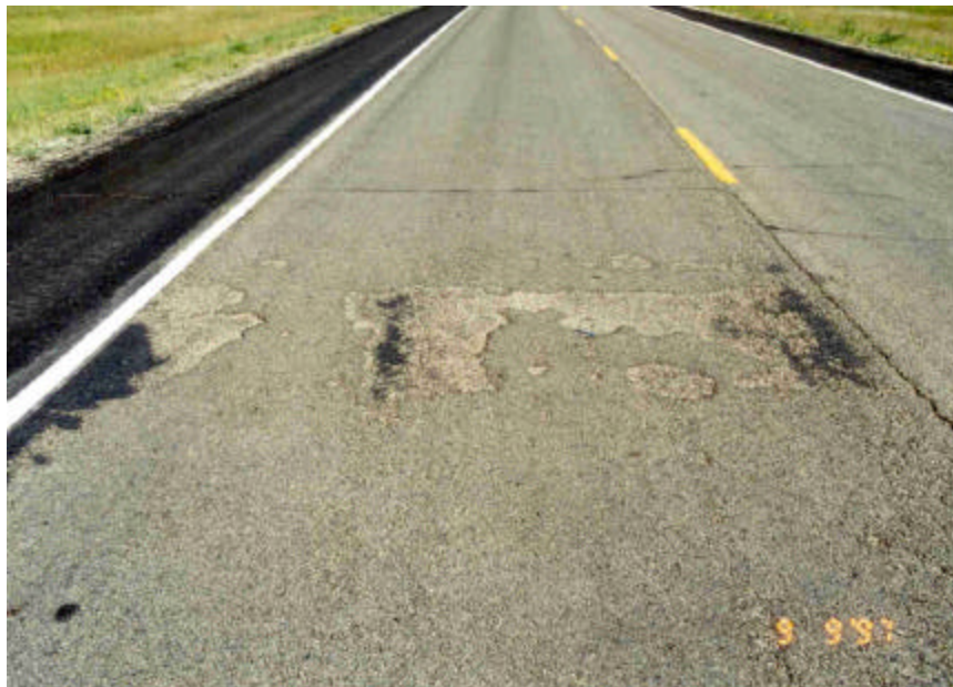
Photo 18 - Typical distress associated with section 7.
