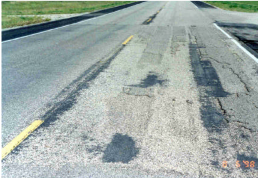
Photo 20 - View of spalled area shown in photo 19 during the summer of 1998.
