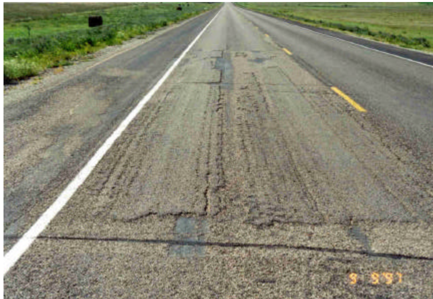
Photo 19 - Large spalled area near the end of section 7 taken during the summer of 1997.
