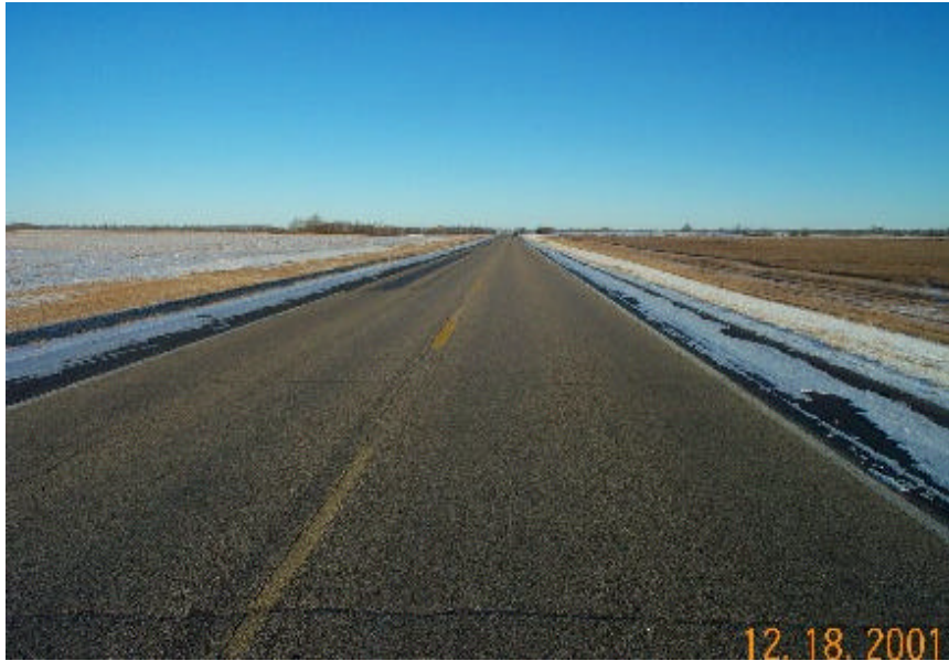
Photo 24 - Overview of section 8. The bleeding in section 8 is the result of a scotch patch, not the original chip seal.
