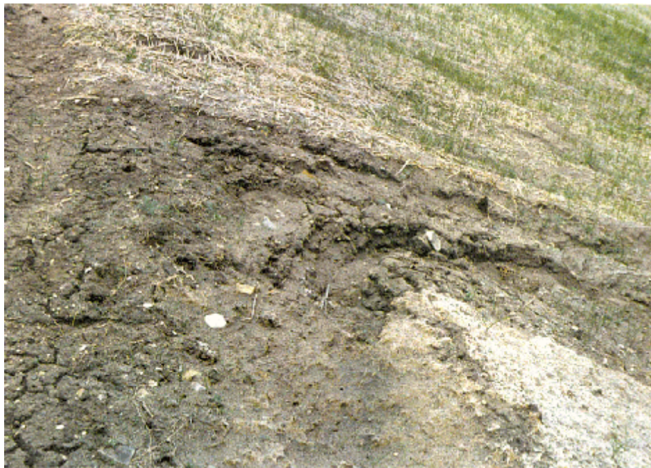
Photo - 14 A view from the top of the slope with the Double Netted Straw on the top of the picture, the narrow strip of uncovered soil in the center and the Soil Guard® on the bottom.
