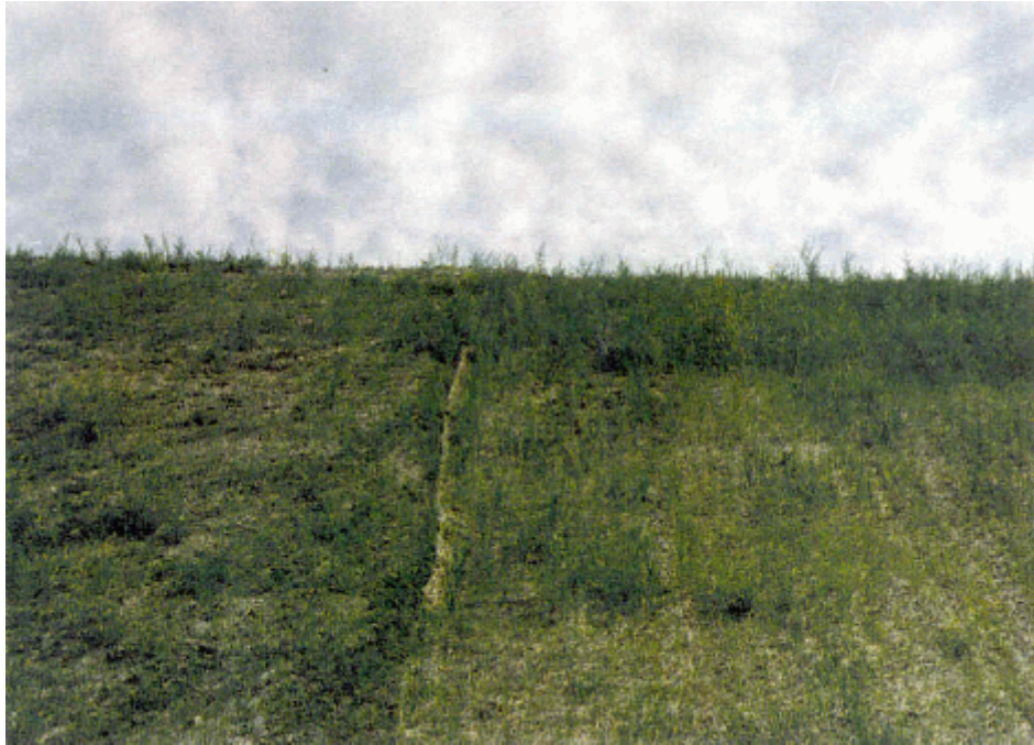
Photo - 19 A view from the bottom of the slope with the Double Netted Straw on the right side of the picture and the Soil Guard® on the left side of the picture.
