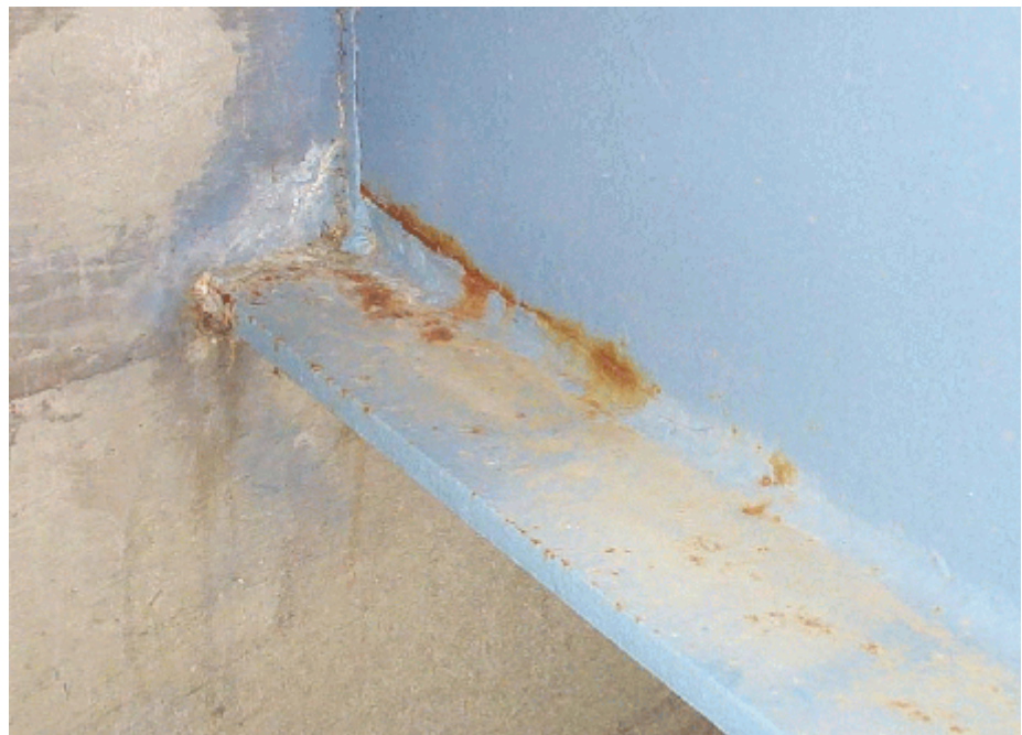
Photo 17: Damaged south beam on westbound structure.
