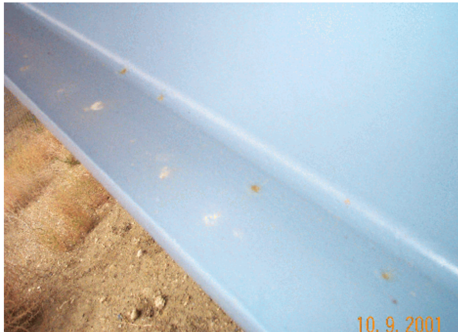
Photo 16: Spot rusting on south beam on westbound structure.
