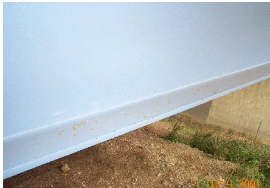
Photo 18: Staining associated with rusting on eastbound structure.
