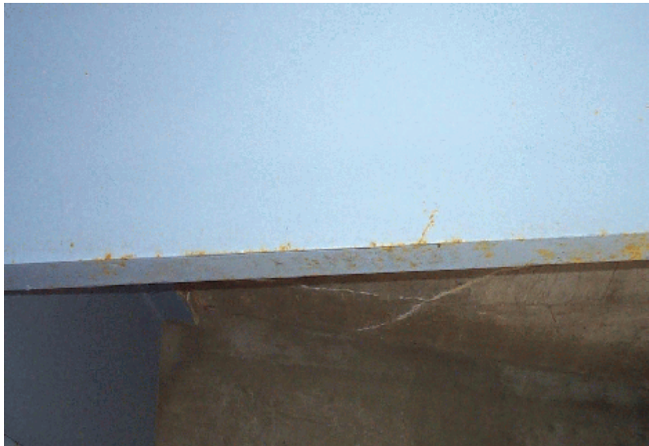
Photo 19: Staining underneath the beam on eastbound structure.
