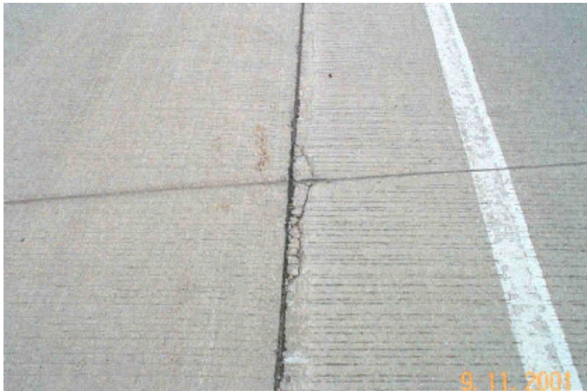
Photo 4. Typical Pavement distress (Sta. 2004+75L).
