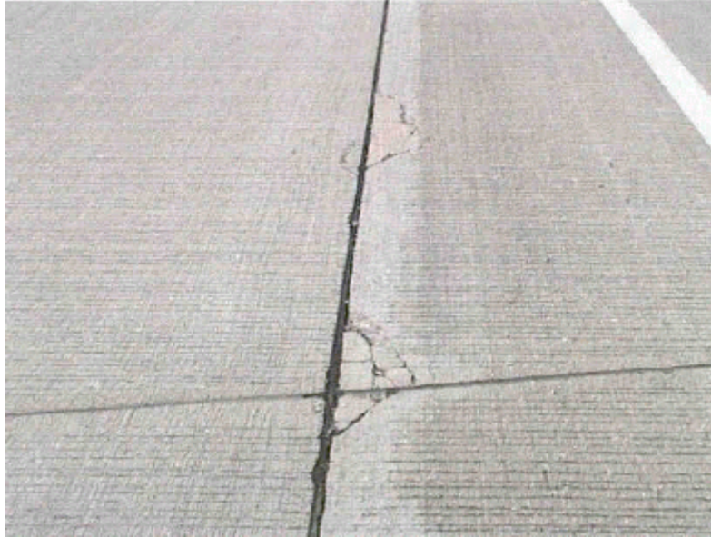
Photo 2. Typical Pavement Distress (Sta. 2160+60L) . Note the snowplow marks on the shoulders.
