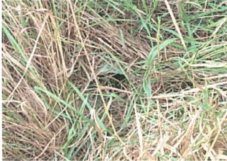
Photo 5. Headwall missing (Sta. 1875+35L).
