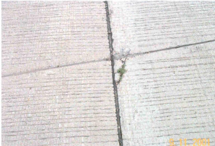
Photo 6. Typical Pavement Distress (Sta. 1875+35L).
