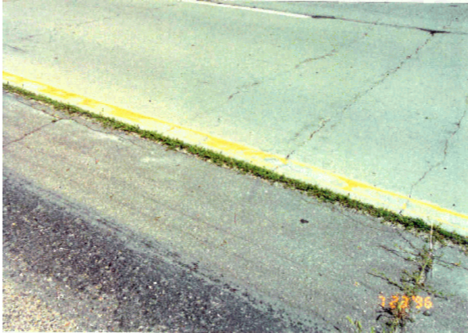
Photo 8. View of the isolated damage on the yellow edge line in the northbound test section between the 12th Avenue North interchange and the 19th Avenue North interchange.
