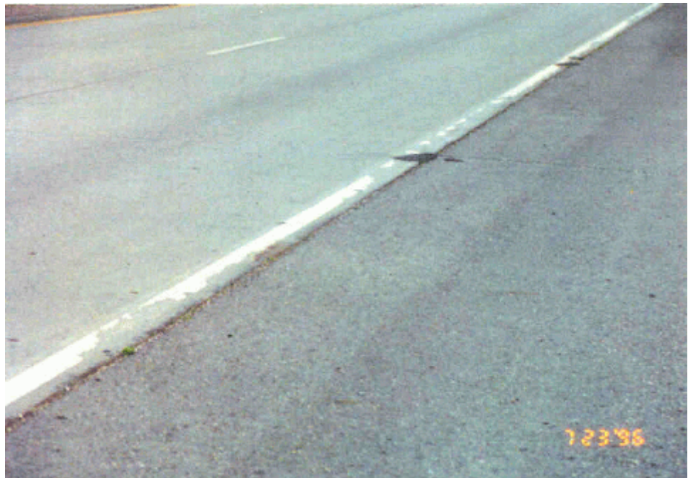
Photo 1. View of damaged white edge line in the northbound test section between the I-94 interchange and the 13th Avenue South interchange.
