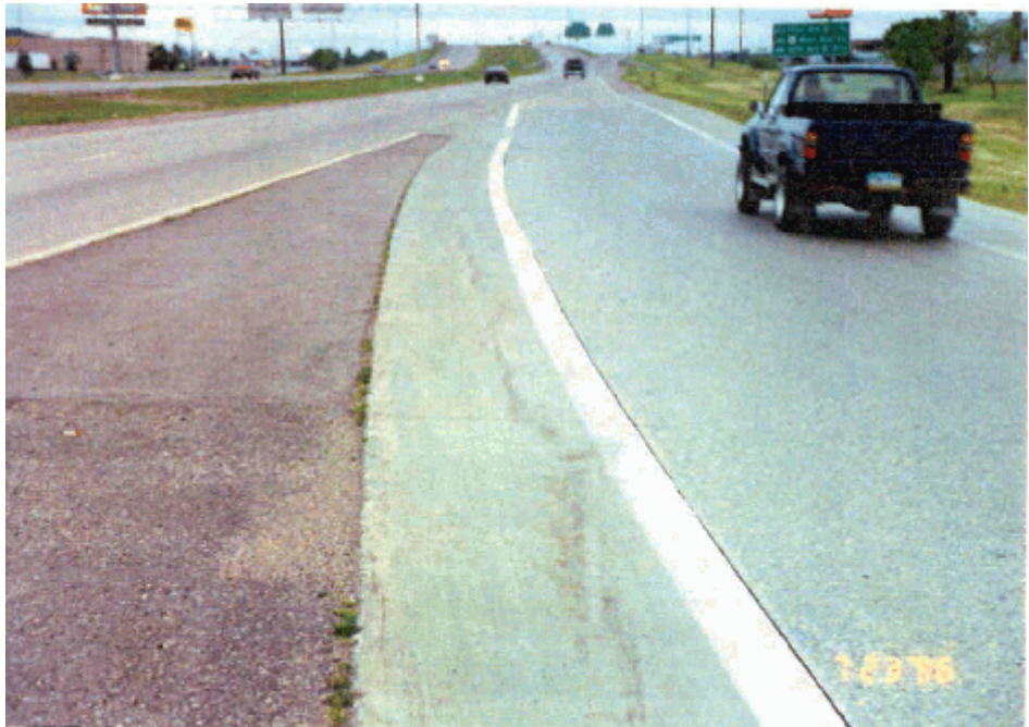
Photo 9. Damaged areas encountered on the northbound on-ramp from I-94 to I-29.
