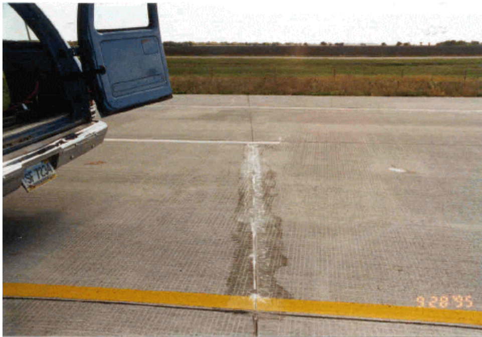
Photo 9. Severe leakage of joint at Station 1094+95
