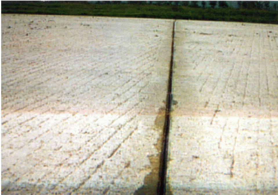
Photo 12. Failing neoprene seal
