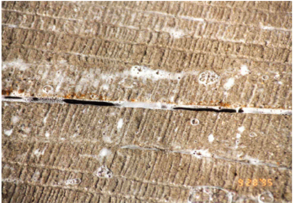
Photo 7. Series of small leaks in station 1135+00
