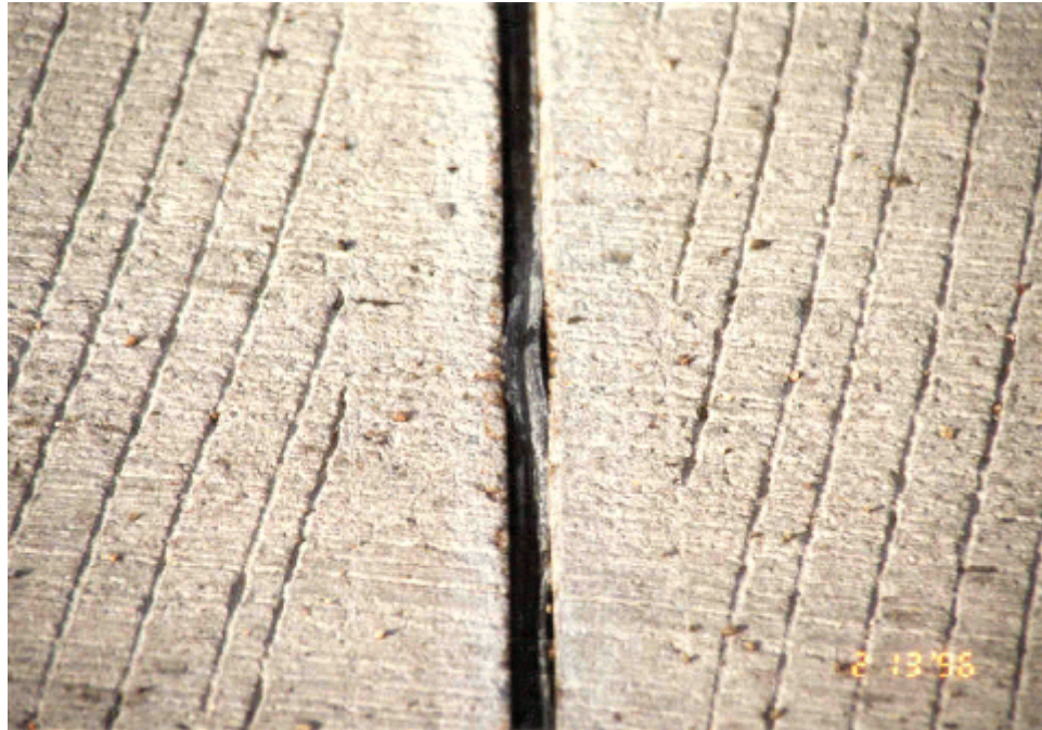
Photo 13. Close-up view of failing neoprene joint
