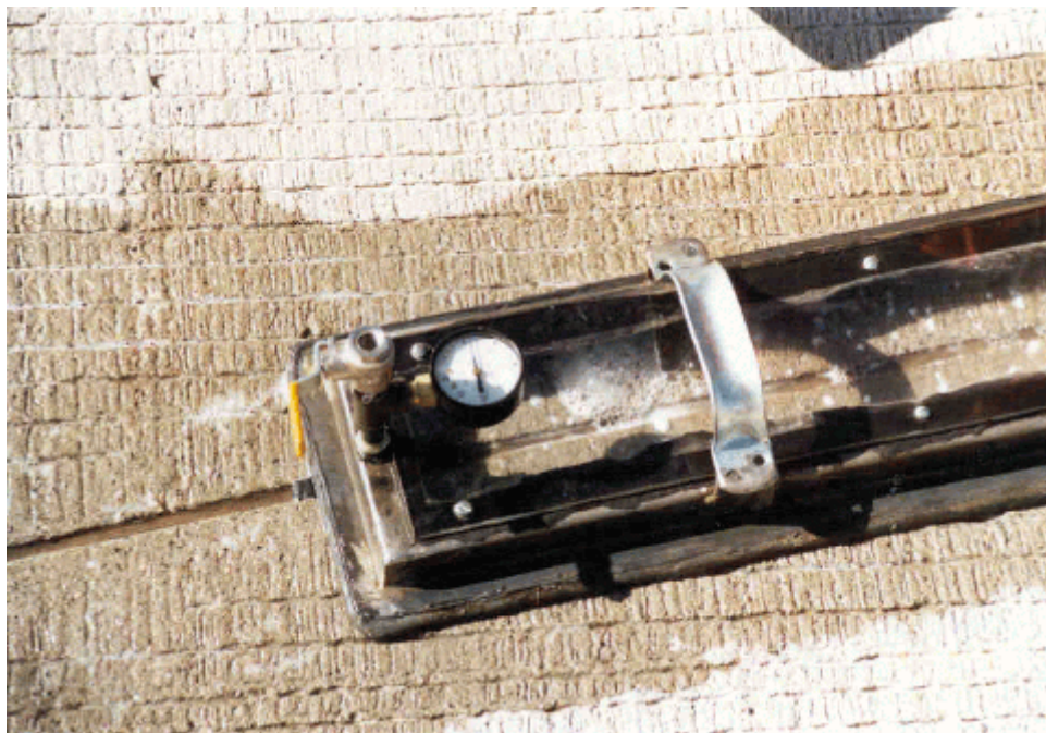
Photo 15. Leakage depicted in silicone sealed joint
