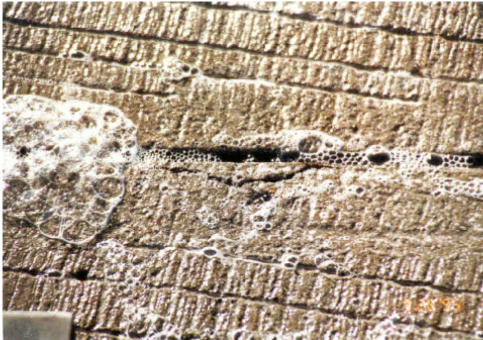
Photo 16. Spall related distress in a silicone sealed joint.
