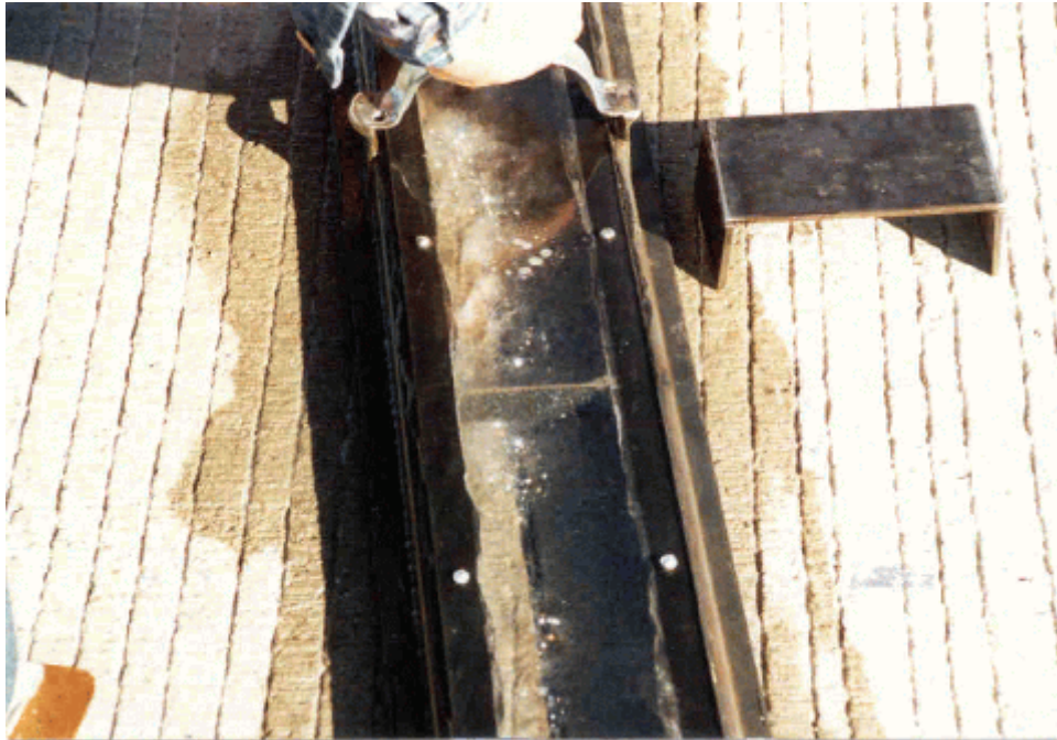
Photo 5. Leaks depicted through window of IA-VAC
