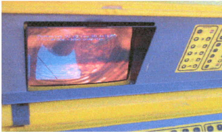
Photo 3: Aggregate blockage in drain pipe.
