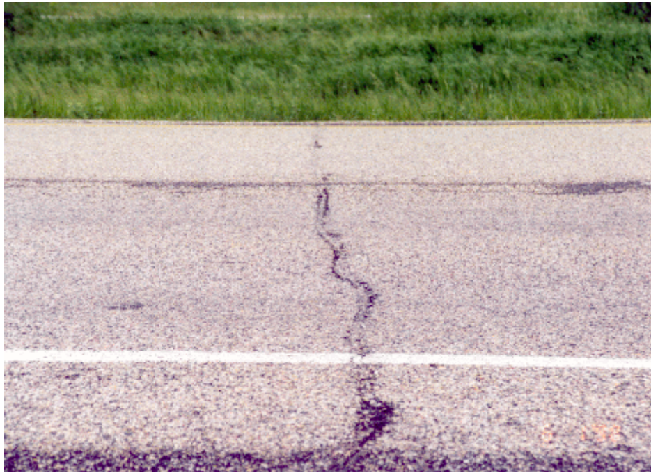
Photo 9 --PavePrep section--typical reflected joint crack--sta.1221+0.6
