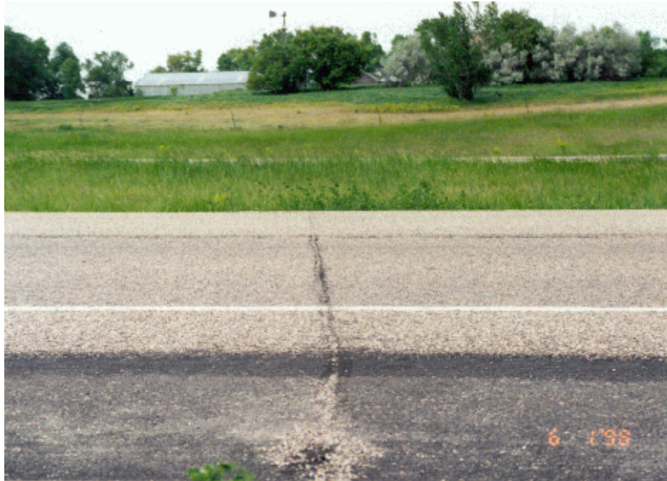
Photo 8 --Control section--reflected joint crack--sta.1213+23.9
