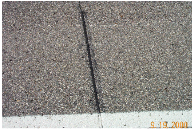
Photo 11 Non squeegeed joint
