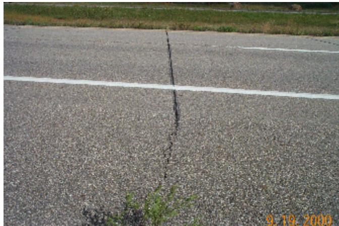
Photo 9 Typical saw and seal crack
