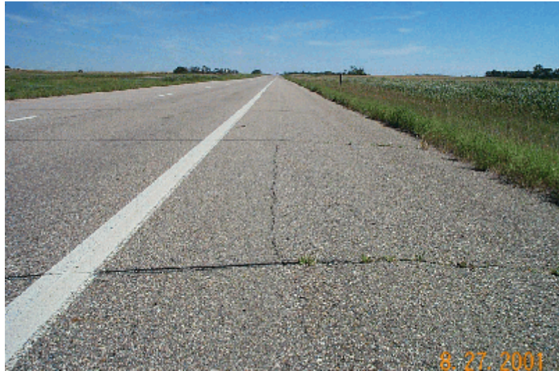
Photo 12 Longitudinal shoulder crack
