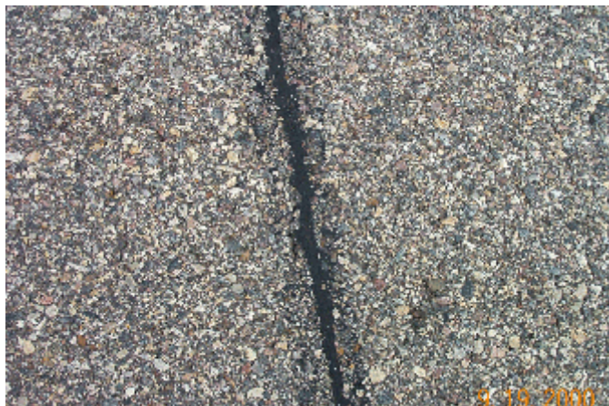
Photo 10 Spalling in wheelpath
