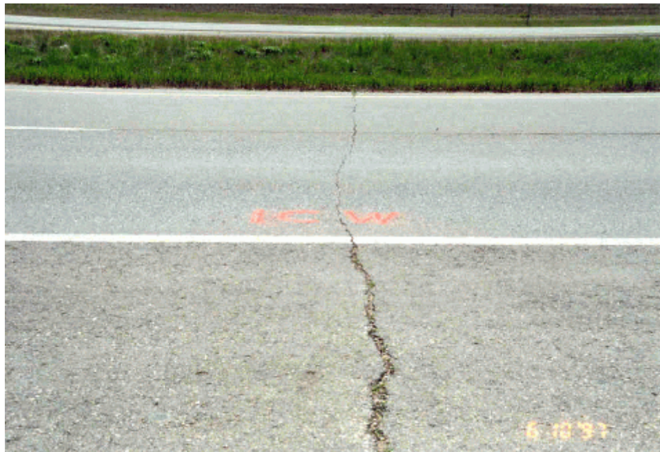
Photo 24. A view of a typical crack in the west control section.
