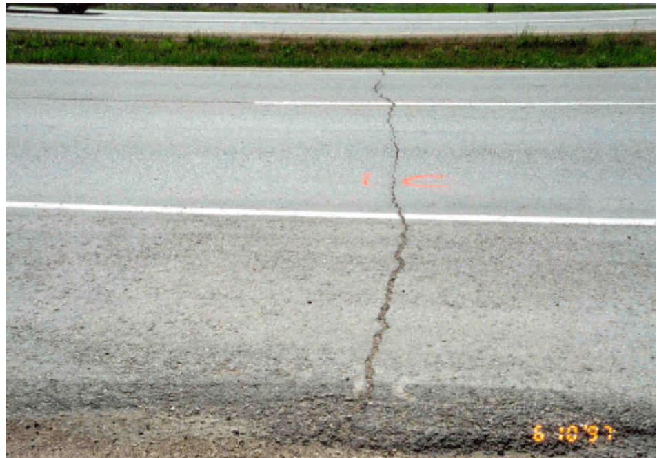
Photo 22. A view of a typical crack in the east control section.
