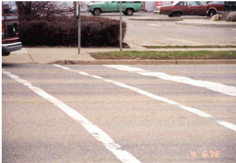
Photo 5. Bismarck Expressway --rutting at stop-bars at 9th St.--W.B.
