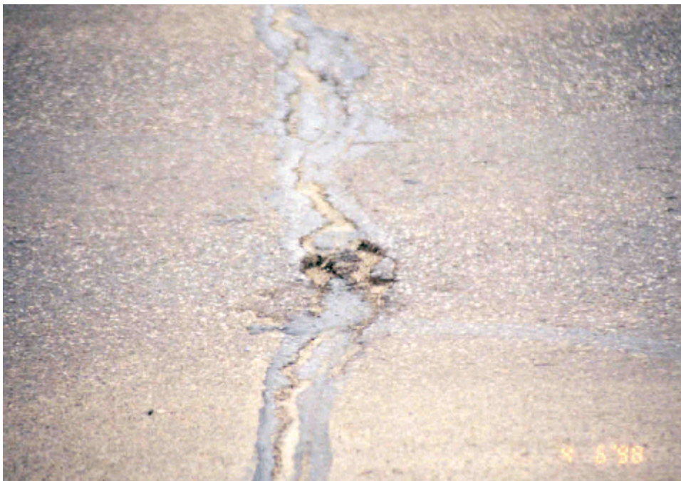
Photo 7. Spalling has resulted in the lost of Ralumac material
