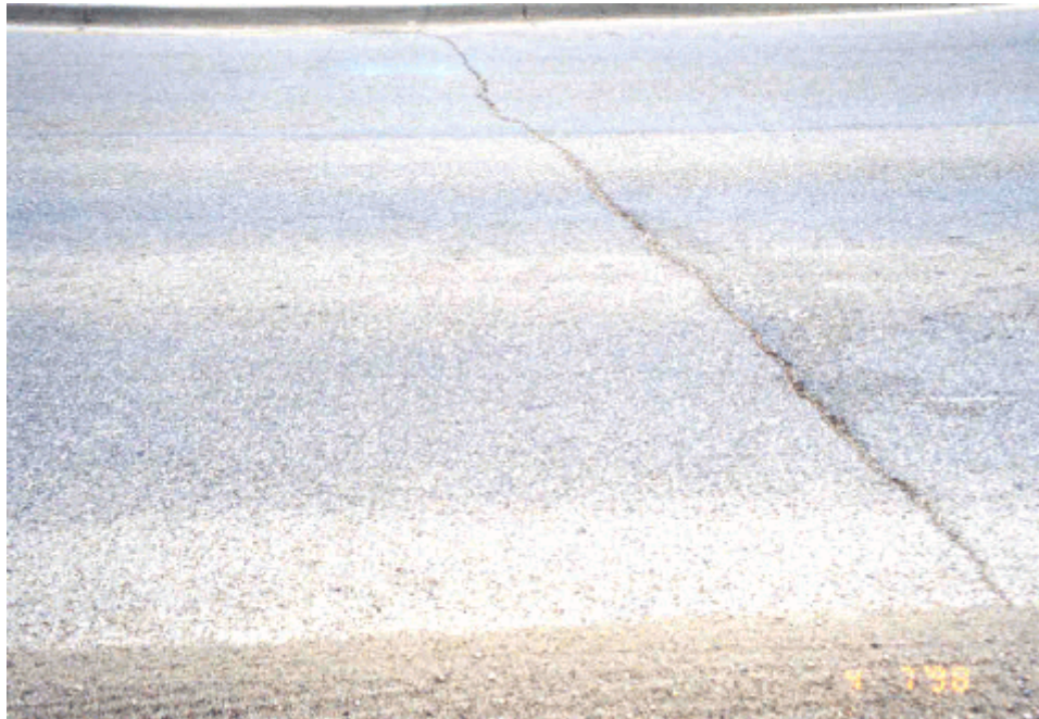
Photo 8. Present texture of Ralumac -- wheelpath and between
