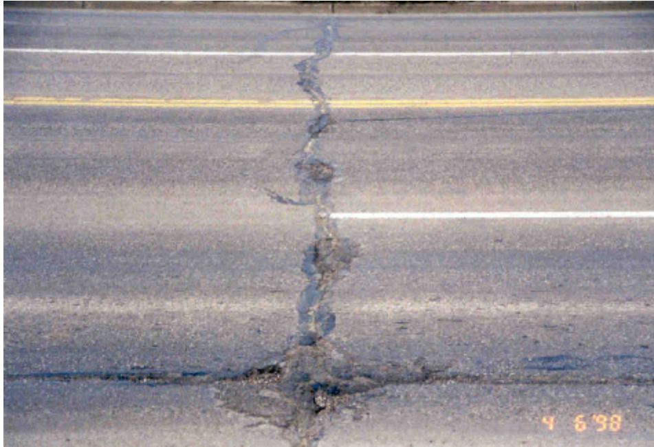
Photo 6. Typical transverse crack ---patched
