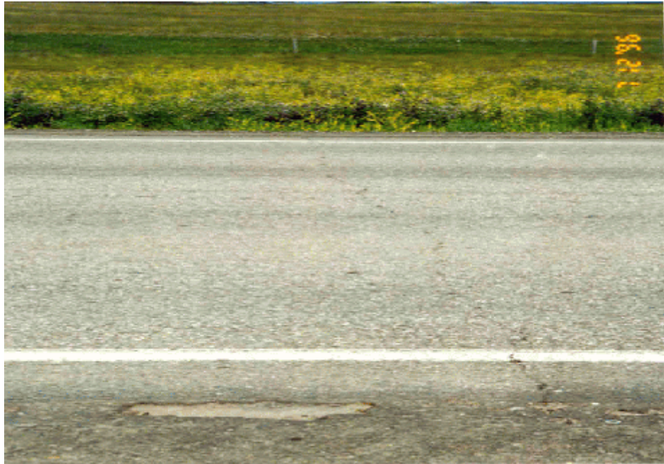
Photo 6: View of crack in control section
