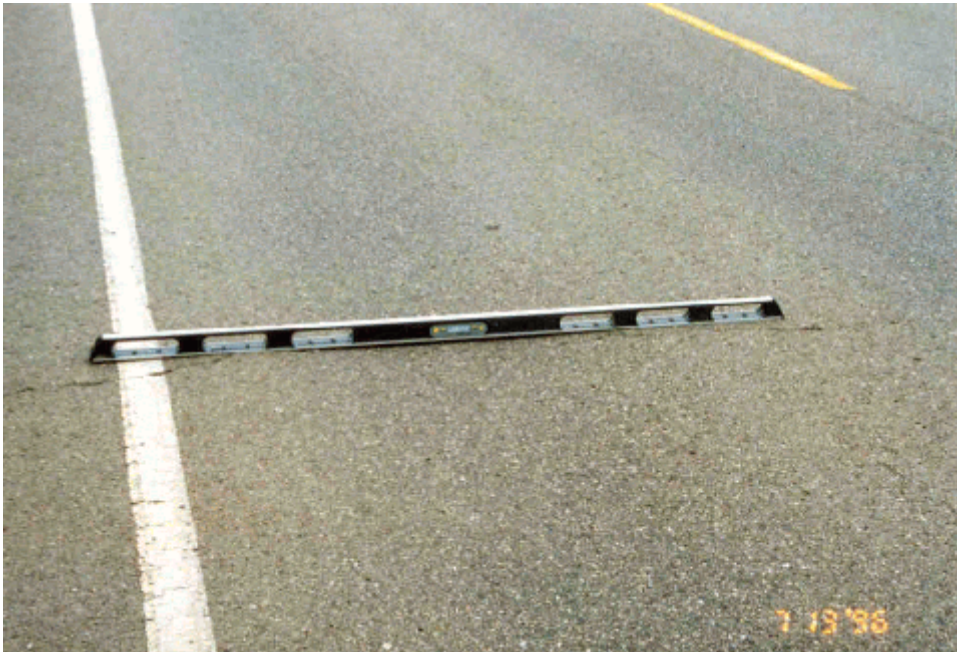
Photo 5: View of rutting in control section
