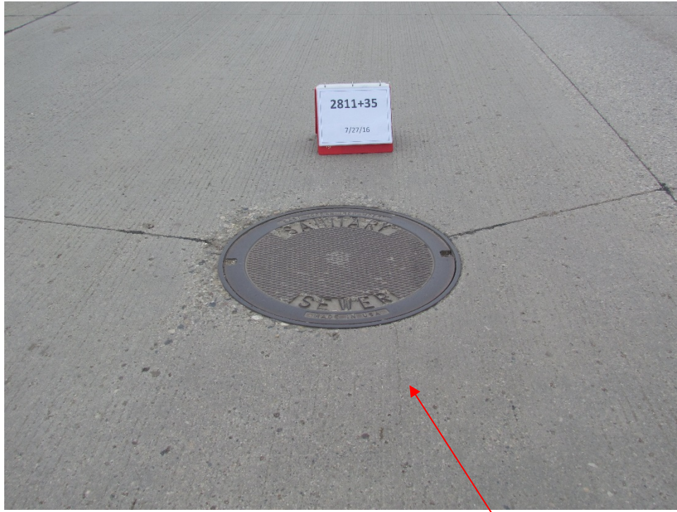
Photo 19: 2811+35 performance evaluation 7/27/16, Hairline Crack Present.
