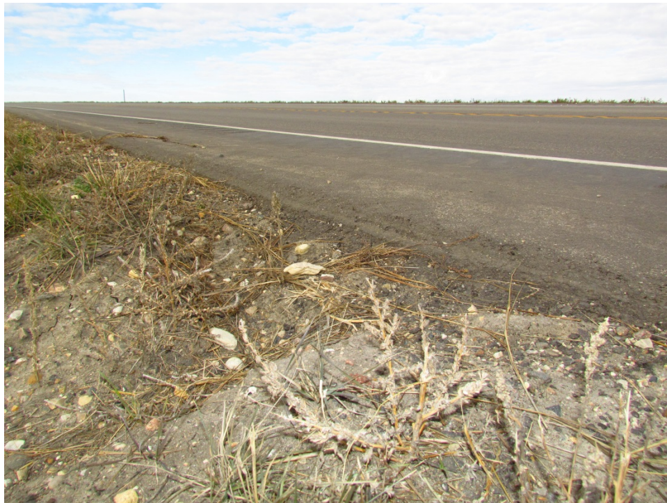
Photo 136: (ND 46, RP 13) - 30° Safety Edge South Shoulder Localized Riling on Super-Elevation
