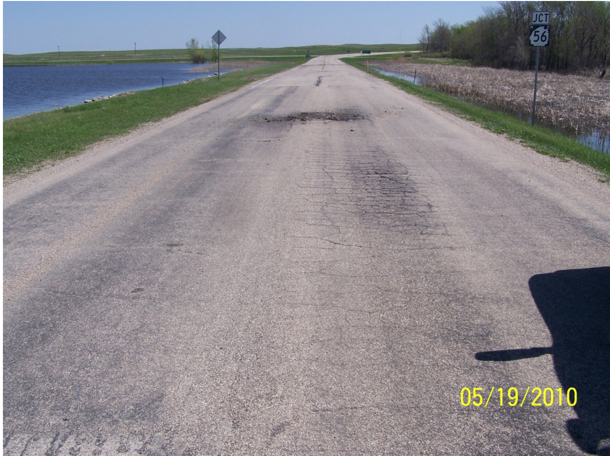
Photo 1 – Severe distresses on roadway near RP 56
