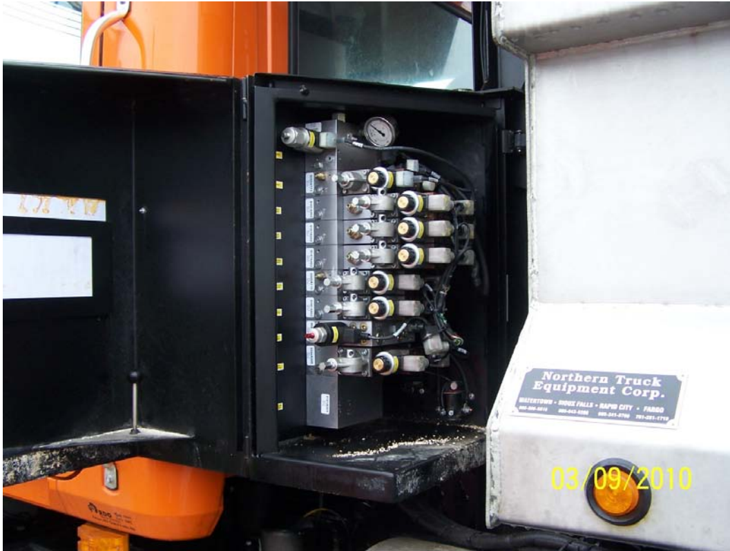
Photo 3 – Hydraulic valves required restructuring to have truck work with TowPLow.
