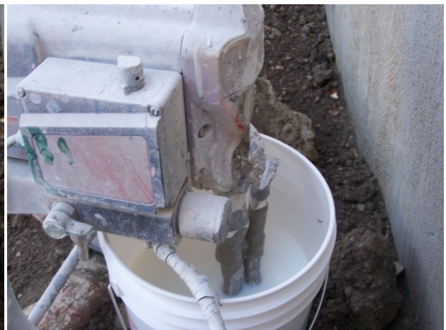
Photo 6: Paint sprayer intake
