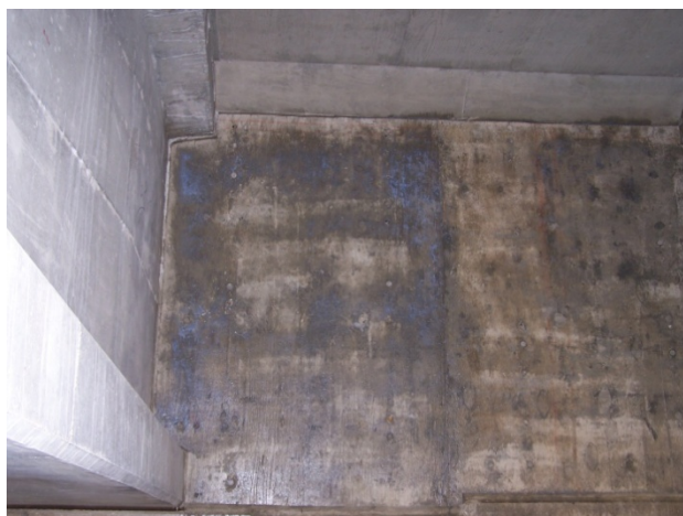
Photo 8: Blue tinted residual moisture
